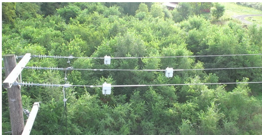
FIGURE 109 3-PHASE LINE SENSOR INSTALLATION
