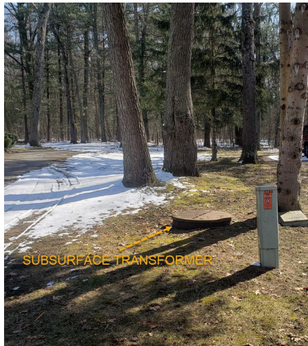
FIELD VIEW OF SUBSURFACE TRANSFORMER
