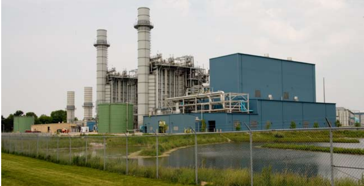
The purchase of the 935-megawatt Zeeland plant helps to fill that gap and meet the intermediate and peak demand needs of its customers.
