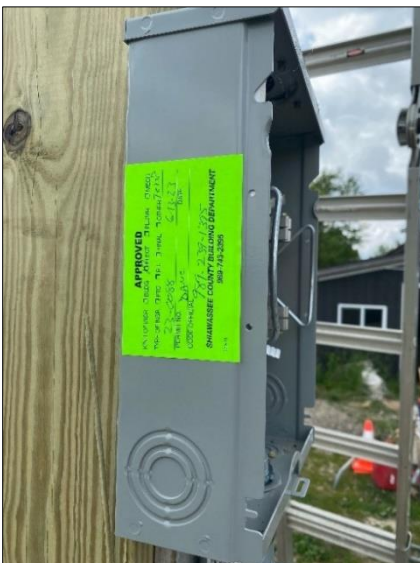
Meter socket inspection sticker.
