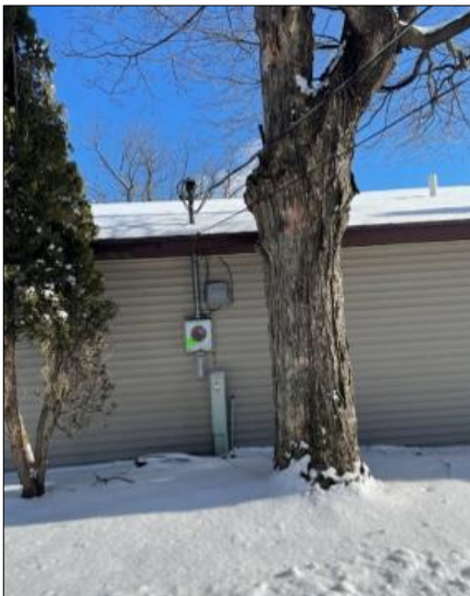
Approved overhead service, meter set only.
