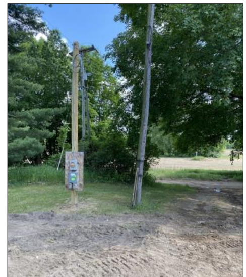
Approved overhead temporary service and a clear path.
