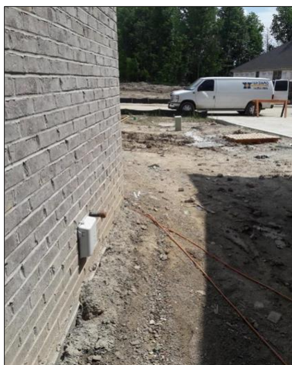
Clear pathway from meter location to the source for direct buried underground.
