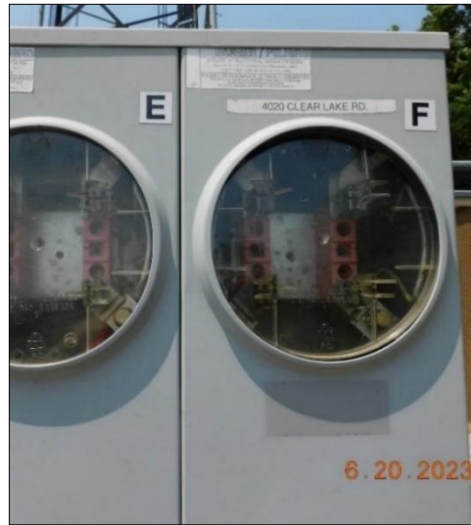
Multiple meter labelling. Meters must be labelled with address or unit number.
