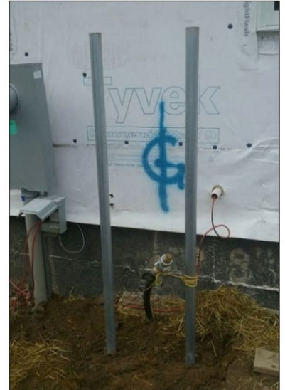
Freestanding/temporary meter post.
