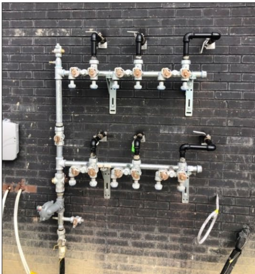
Multi-meter bracket showing Consumers Energy tags on fuel lines and service line connected to bracket.
