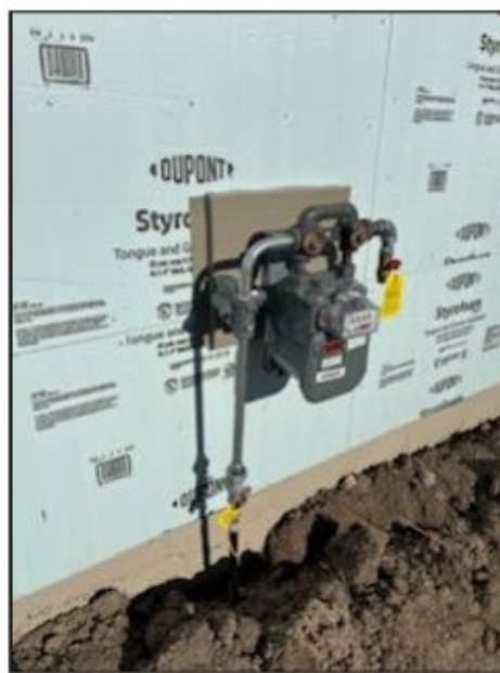
Meter mounted on a weatherproof permanent backer plate.
