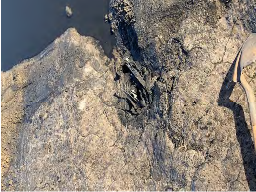
Picture 03 - Visual Identification of Primary Liner Damage – Shovel on the Right for Scale
