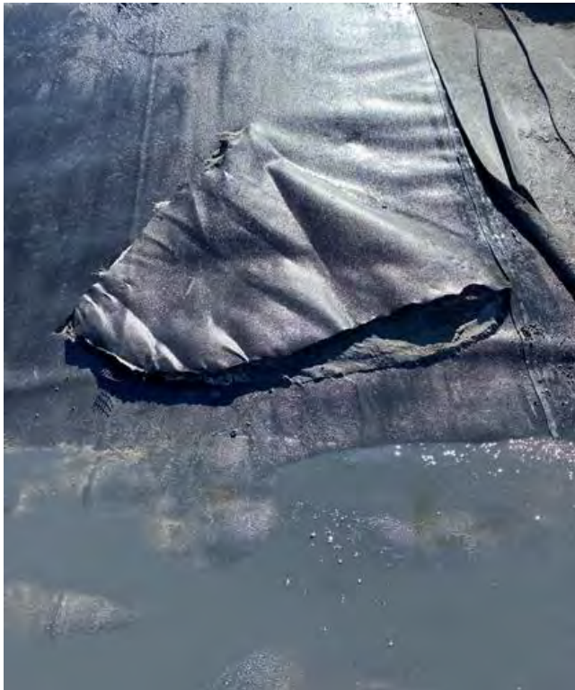
Picture 06 – Observed Damage at Visual Observation Point No. 2
