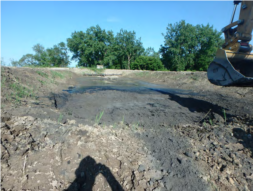
Adding material to Chemical Pond B residual to dry for transport to Pond 1, Looking South.
