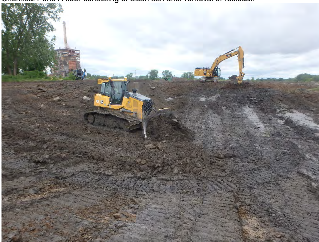
Placing bridging layer of structural fill across floor of Chemical Pond A, Looking North.
