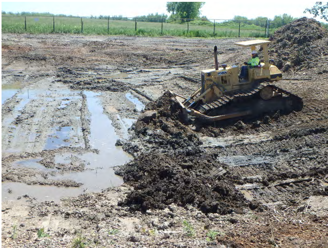
Cutting residual material in Chemical Pond A to dry prior to removal
