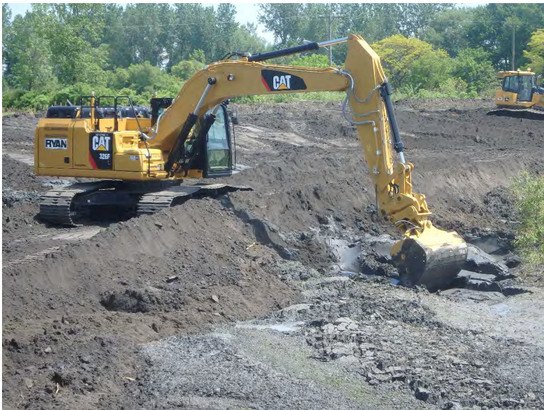
Removing saturated material from floor of Pond 1 prior to placement of bridging layer.
