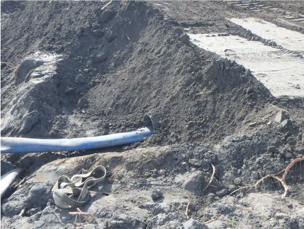
Temporary culvert installed for 6" pump discharge hose under access road between Ponds 1&2.
