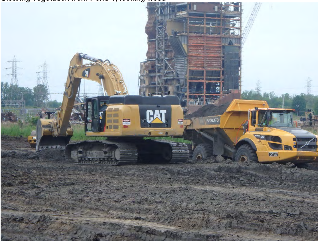
Cutting area north of Chemical Pond B down to structural fill grade, looking west.
