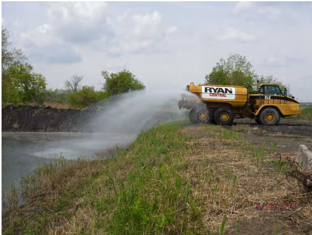
Discharging water from Chemical Pond B via the water truck into northwest corner of Pond 1.
