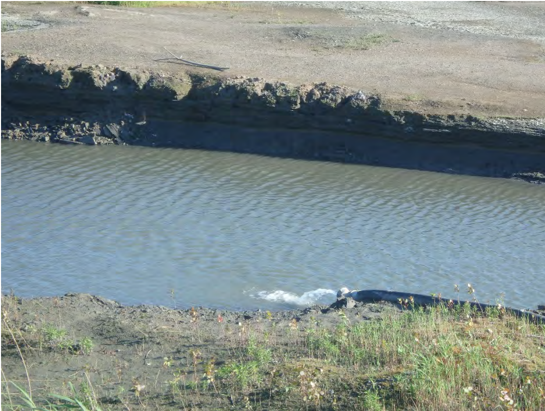
Backflush of filters on Pond 2 dewatering system, looking north.
