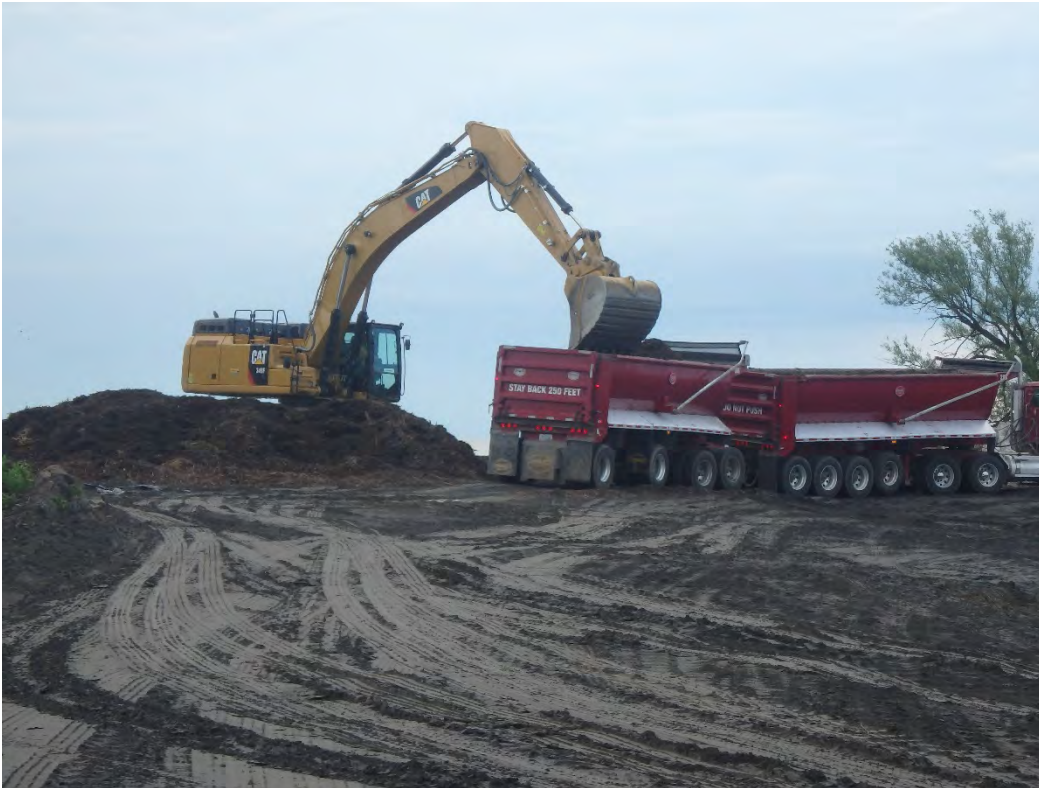
Loading of vegetation chip pile for disposal at offsite facility, looking east.
