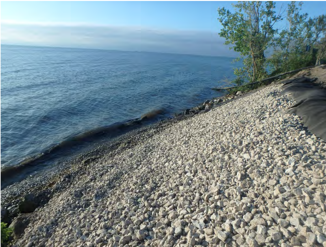
Textile and D50/2 inch cushion layer placed on shoreline southeast of Pond 2, looking south.
