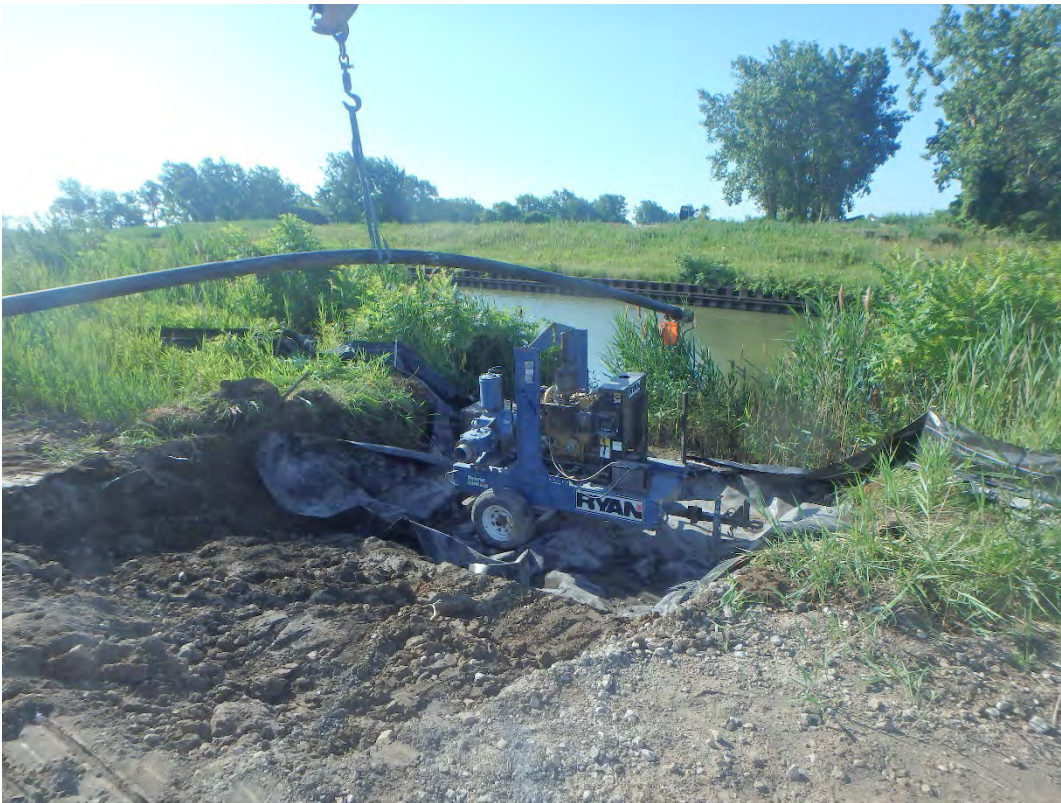
6 inch pump set southwest of Pond 2 along the discharge channel, looking south.
