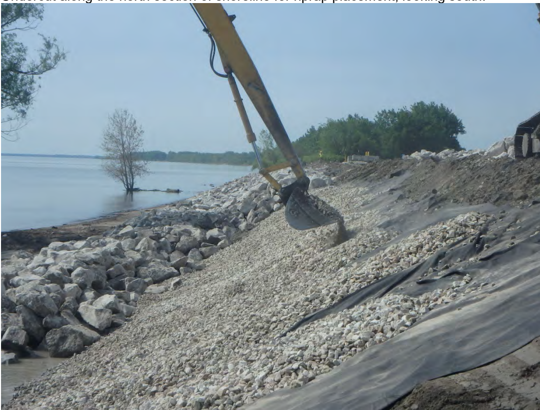
D50/2 inch cushion layer being placed atop textile along shoreline, looking south.
