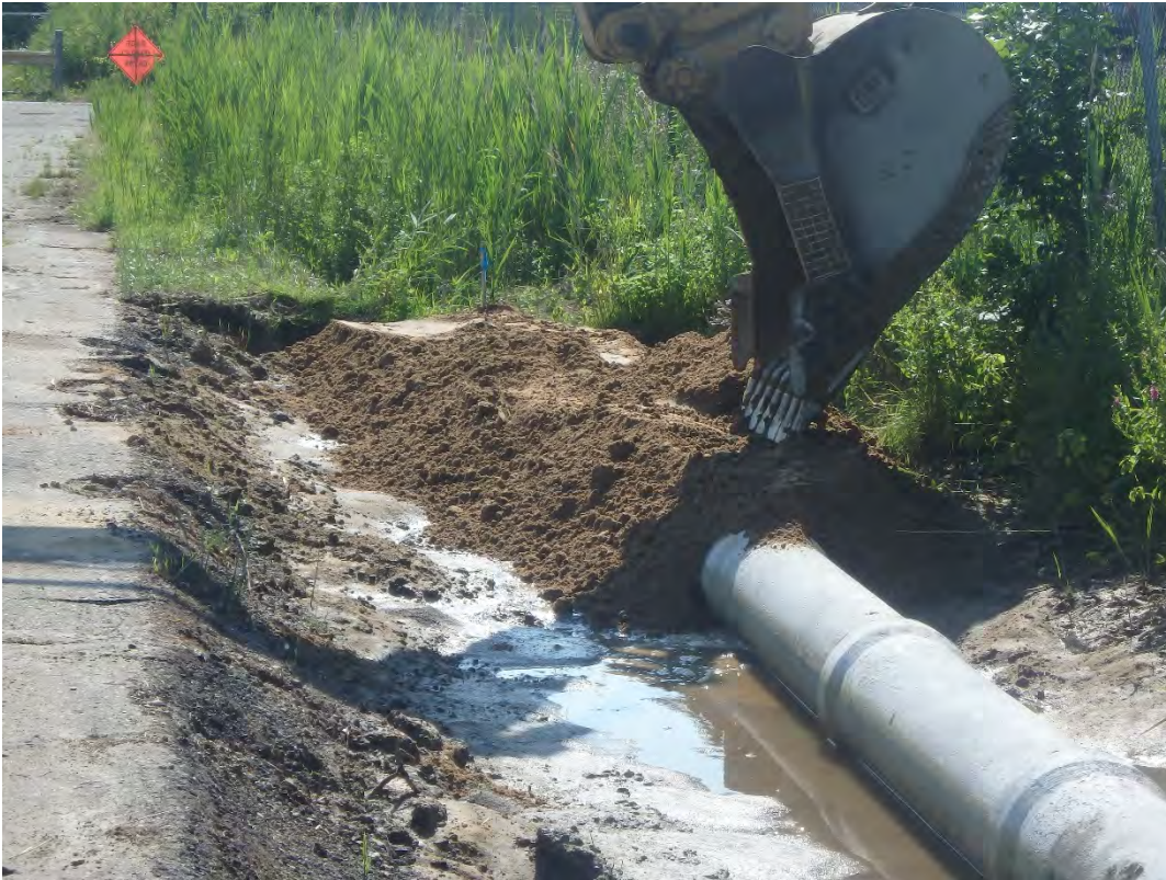
Placement of class IIIA sand for backfill over access road culvert, looking east.
