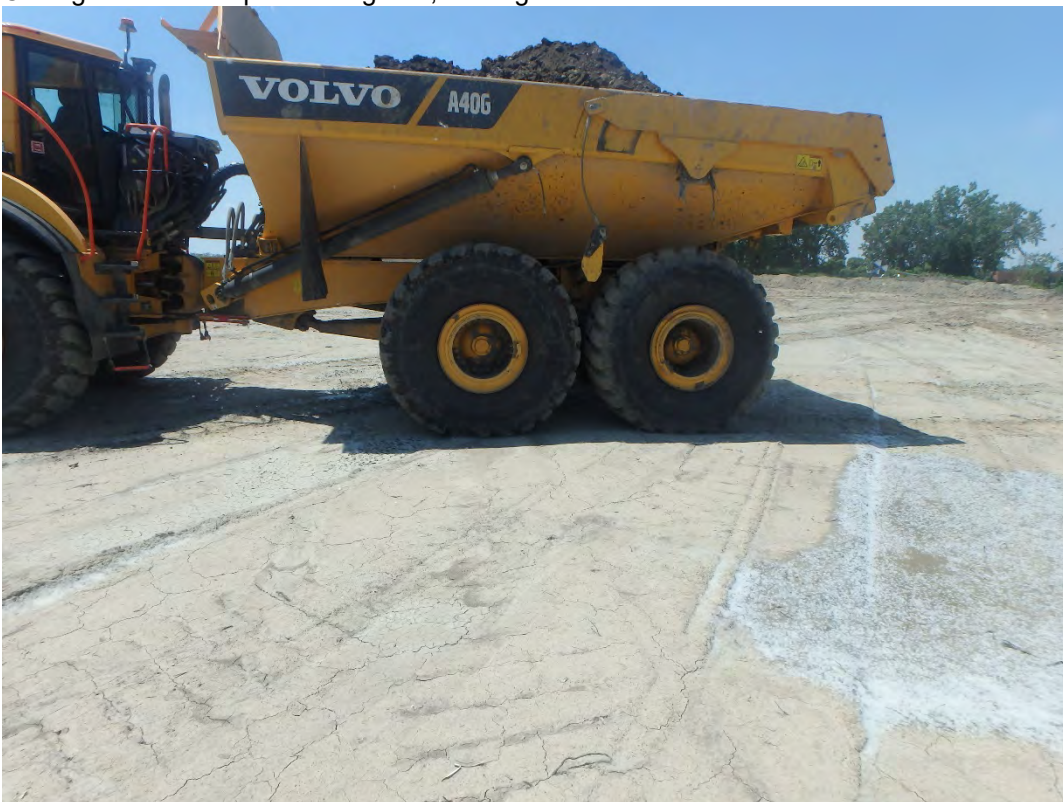
Proof roll of onsite structural fill placed over chemical ponds, looking west.
