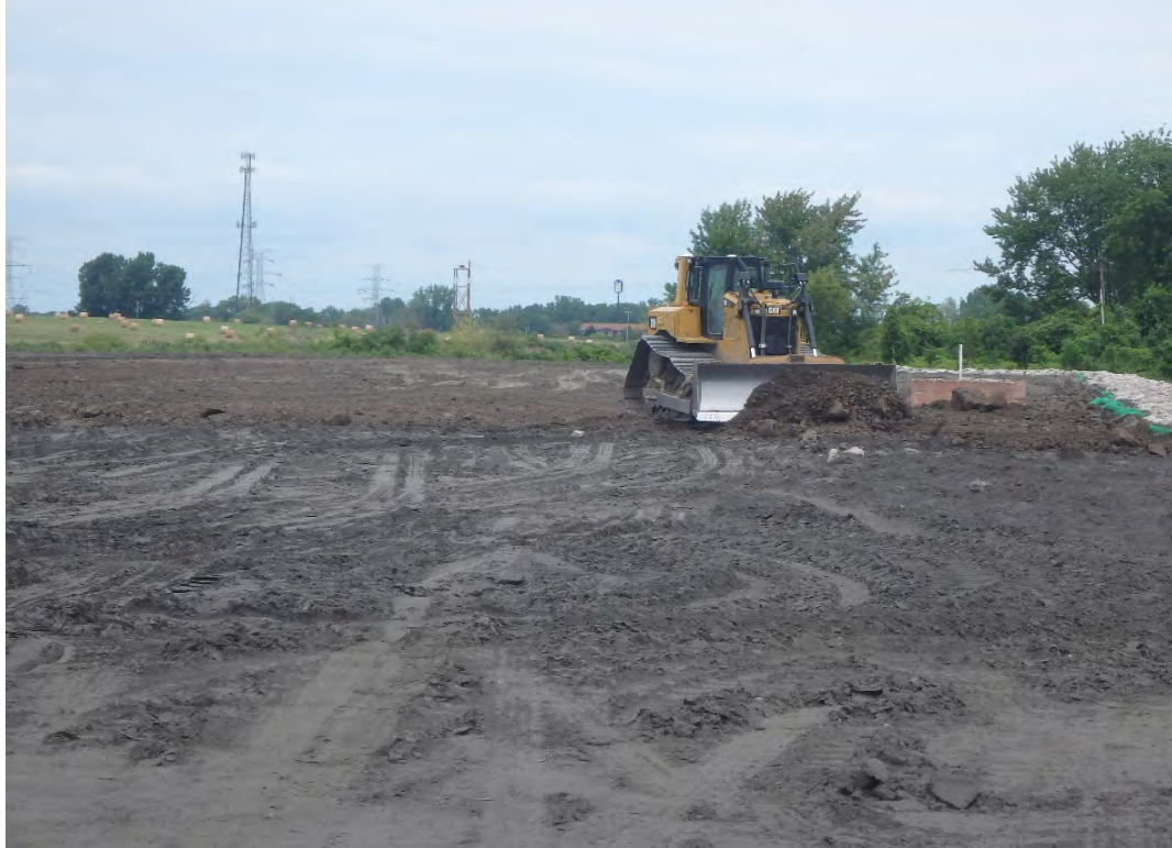
Placing lift of structural fill east of Pond 1 along top of shoreline slope, looking north.
