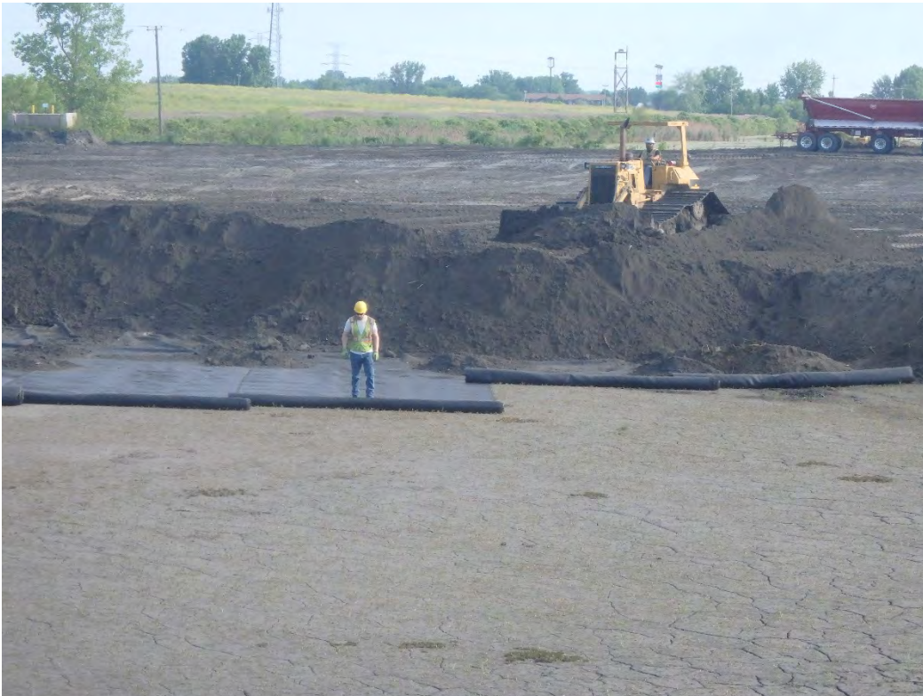
Deployment of geotextile and placement of bridging layer in Pond 1, looking north.
