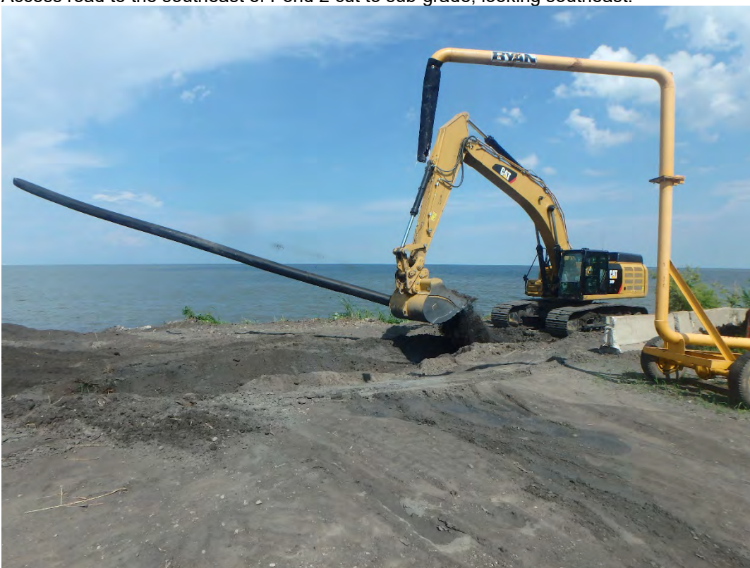
Removing utility pipe running from southeast corner of Pond 2 too Chemical Ponds, looking east.
