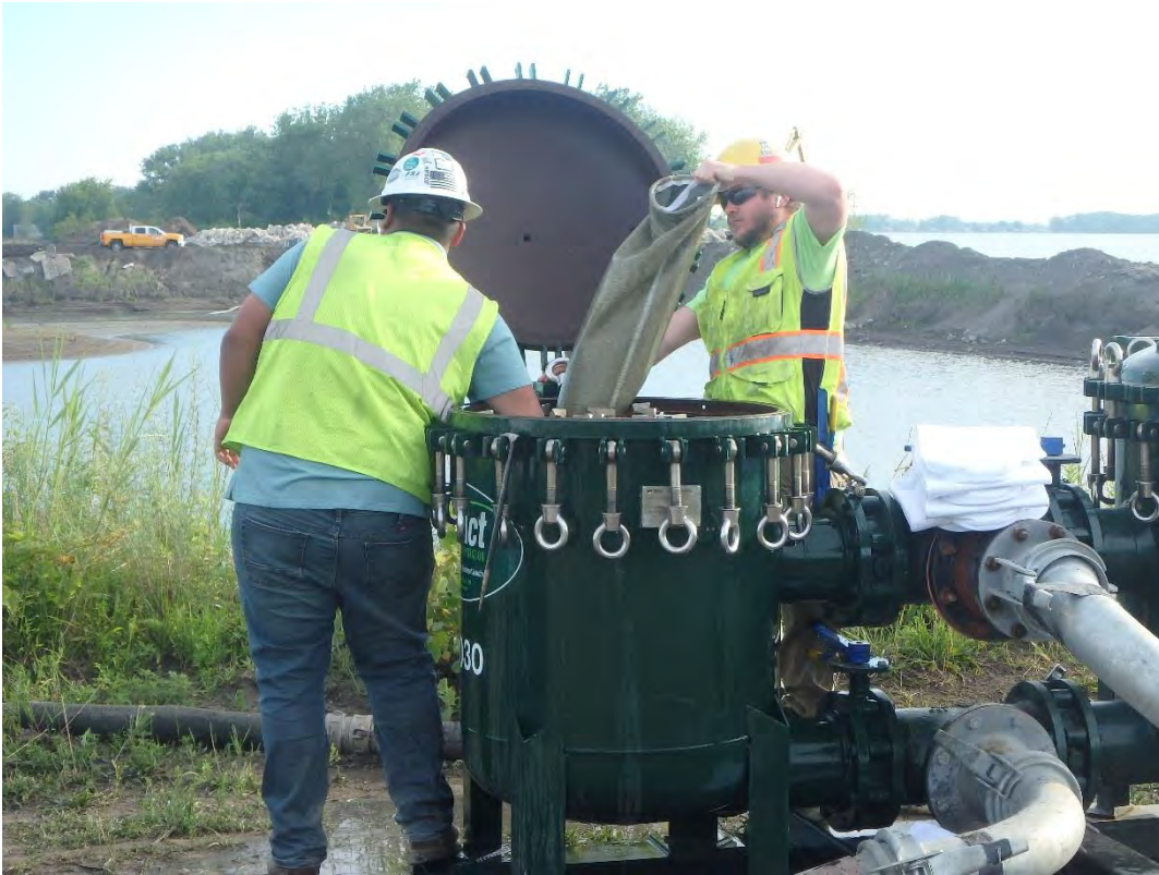
Filter change on the dewatering system for Pond 2, looking northeast.
