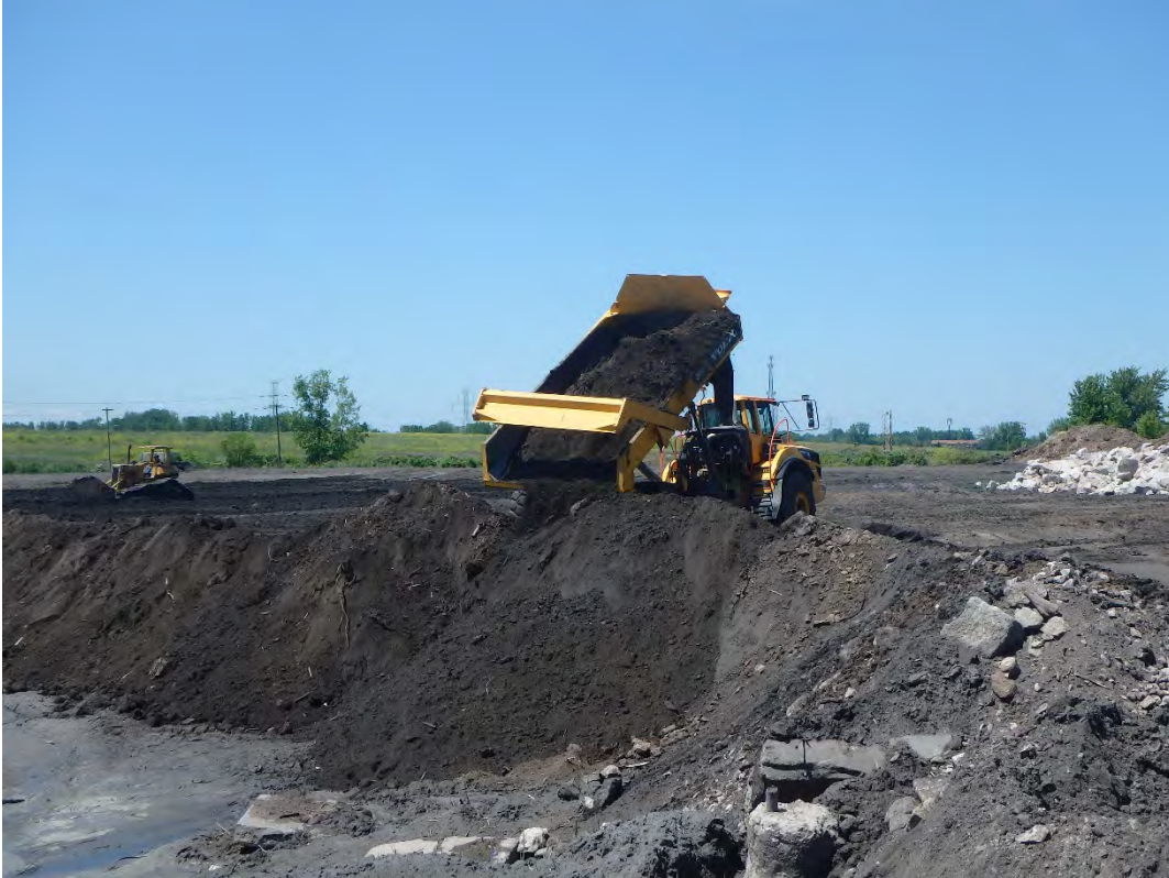
General fill from grading of shoreline being placed into Pond 1, looking north.
