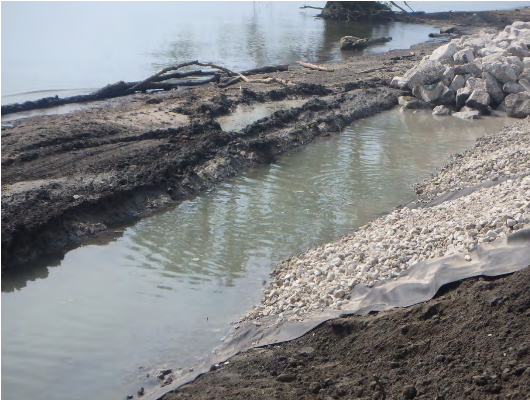
Undercut along the north section of shoreline for riprap placement, looking south.
