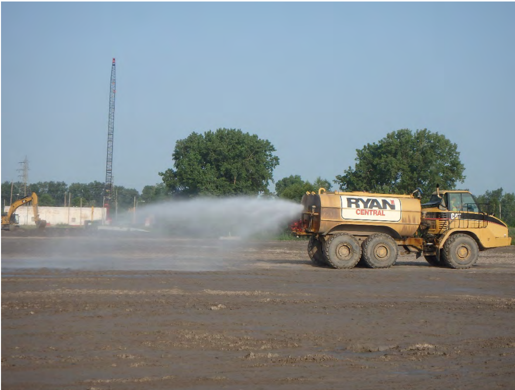
Dust control and moisture maintenance of fill placed in Pond 1, looking west.
