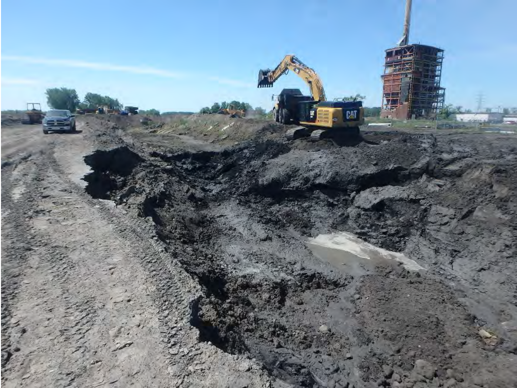
Removal of saturated material from along the west side of Pond 1, looking south.
