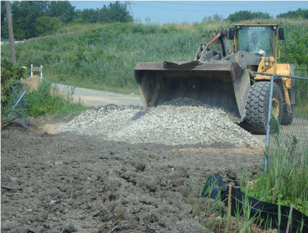
Construction of temporary access road into Pond 1 from Lake Erie RD., looking northwest.
