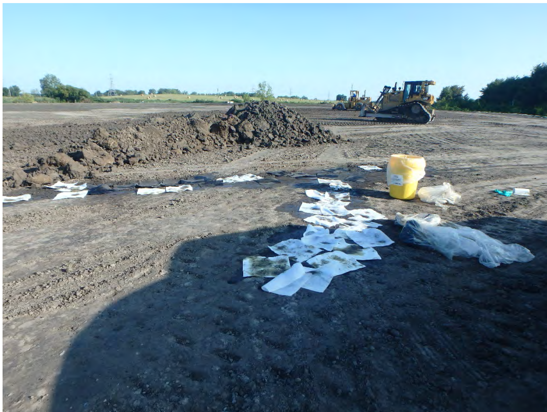
Absorbent pads used for hydraulic oil leak in Pond 1, looking north.
