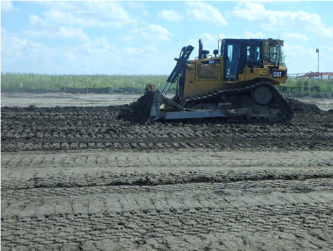
Placement of 12 inch loose lift of structural fill at chemical ponds, looking south.
