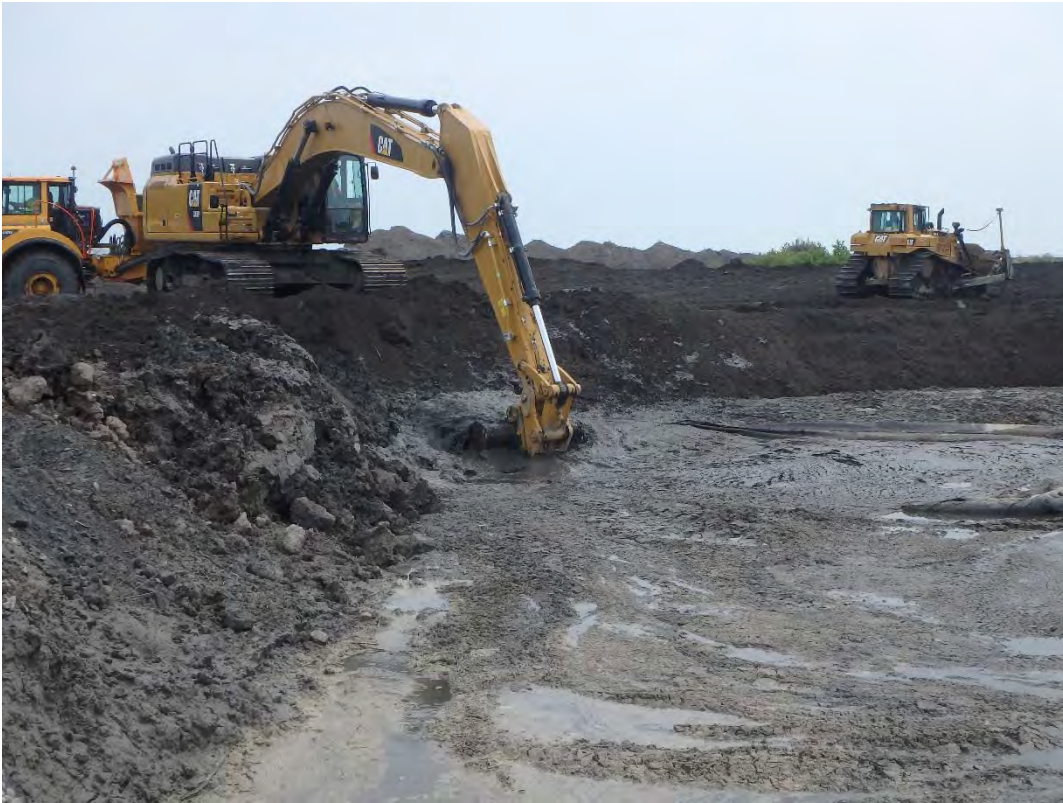
Excavation of saturated material in the northwest corner of Pond 2, looking east.
