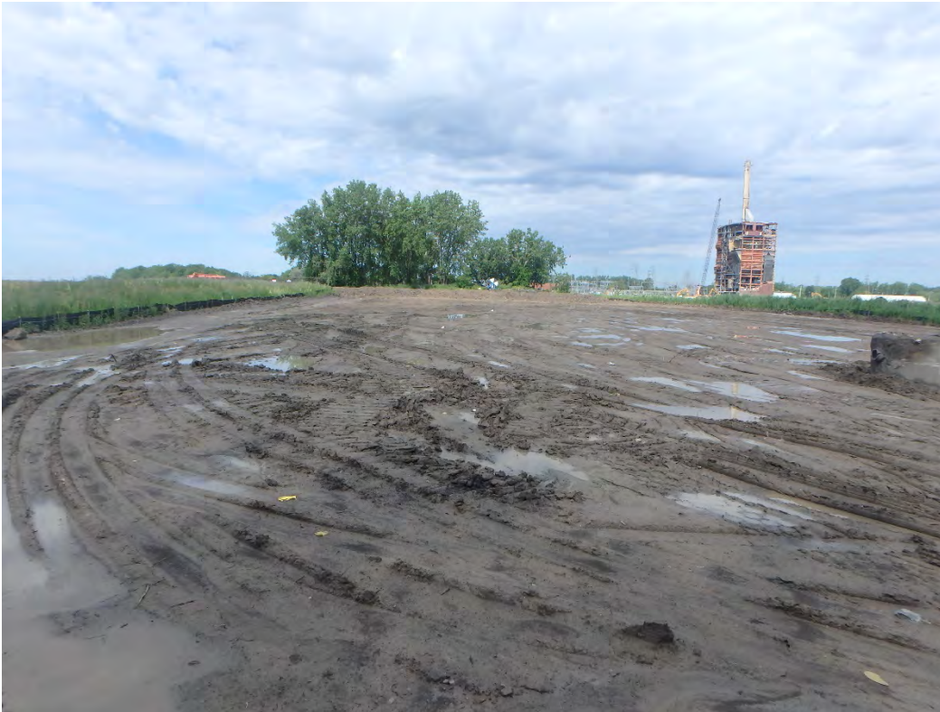
Chemical Ponds 1 st lift of structural fill after previous night's rain, looking west.
