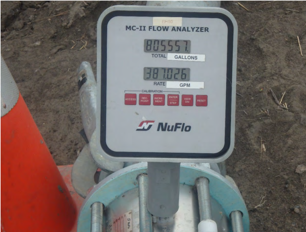
Discharge flowmeter on dewatering system in Pond 2.
