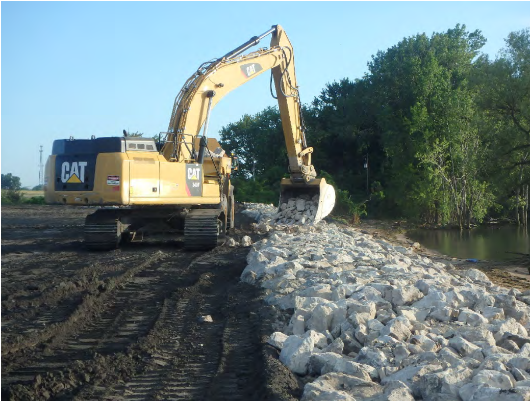
Placing 8 x 16 inch riprap to fill voids in the D50/30 inch along shoreline, looking north.
