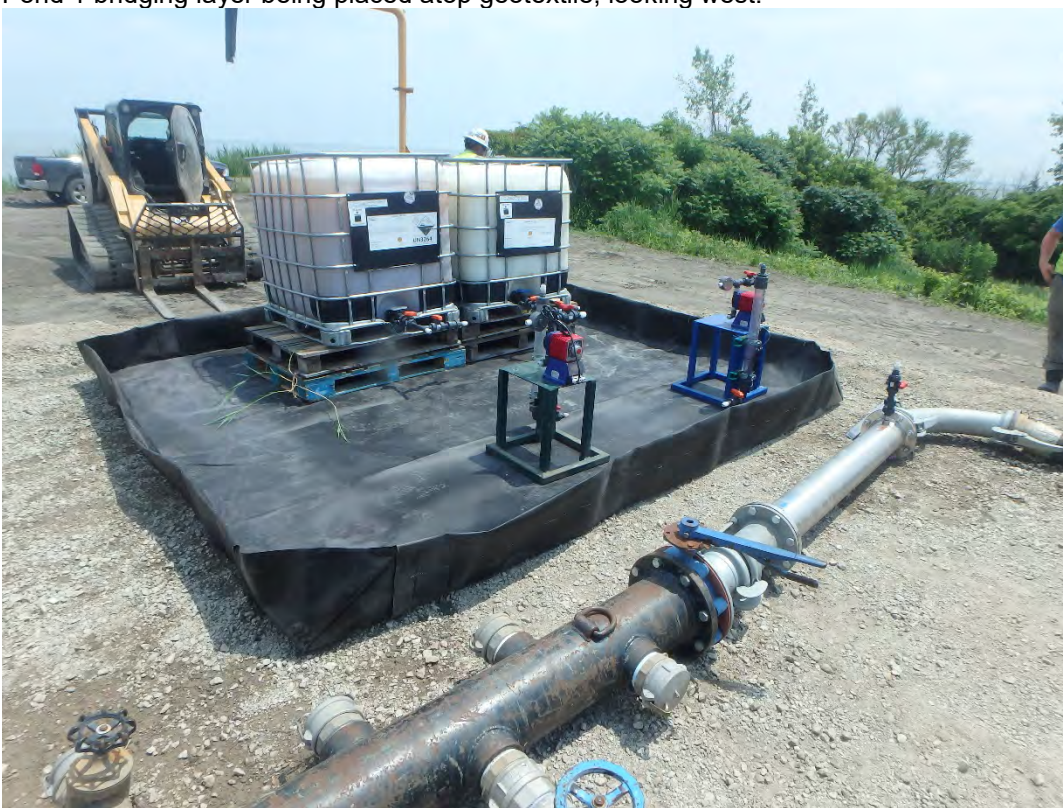
Installing equipment to supply Flocculant to supply side of Pond 2 dewatering system, looking southeast.
