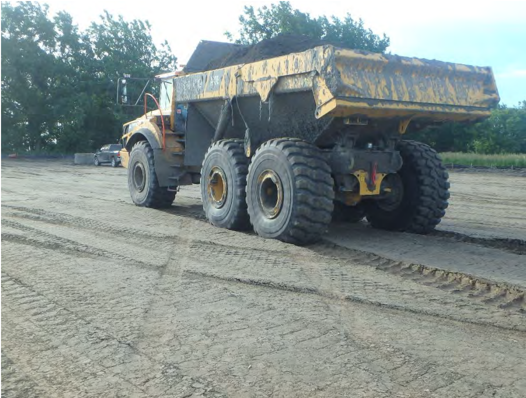
Proof roll of compacted onsite structural fill placed in Chemical Ponds Grading Area, looking west.
