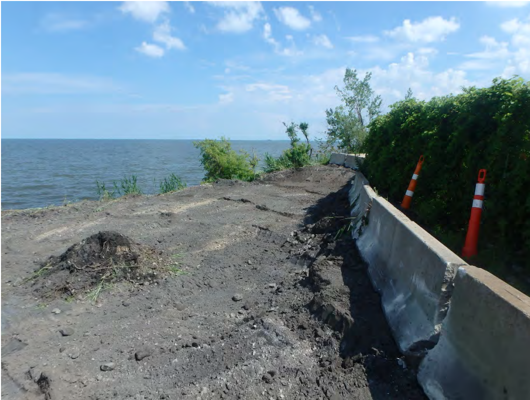
Access road to the southeast of Pond 2 cut to sub-grade, looking southeast.
