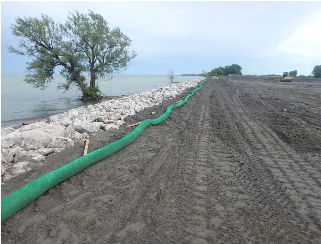
Waddles installed along the western edge of shoreline riprap east of Pond 1, looking south.
