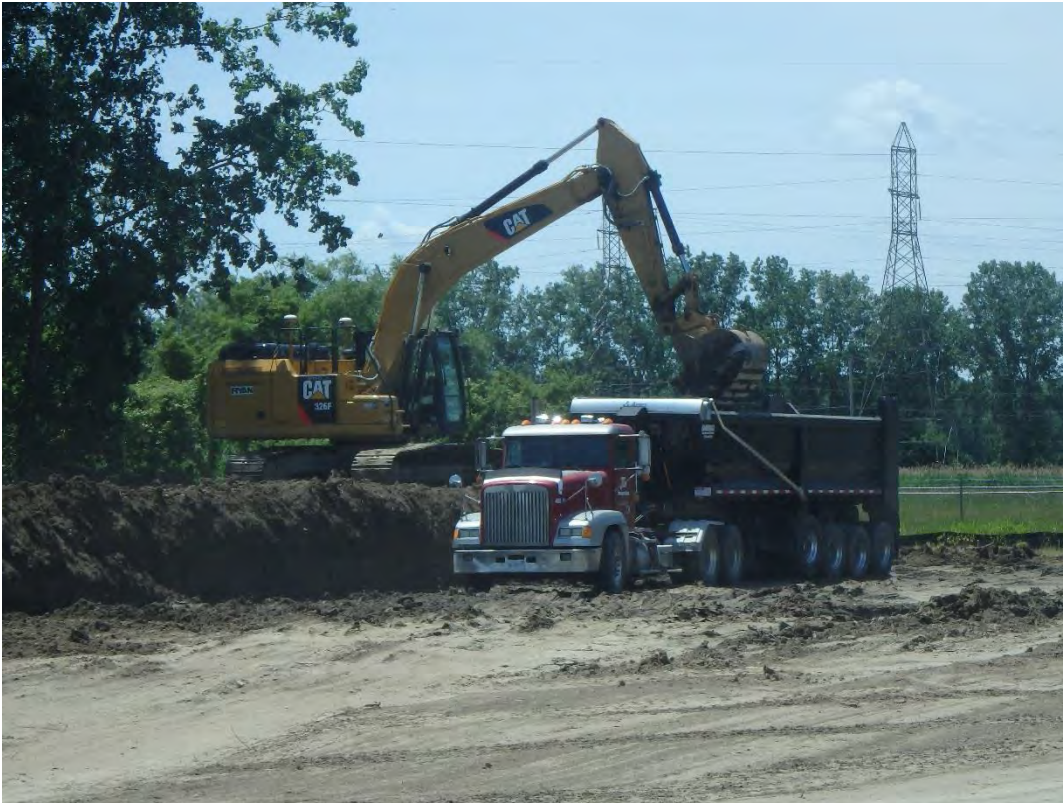
Loading onsite structural fill for stockpiling in the Chemical Ponds Grading area, looking west.
