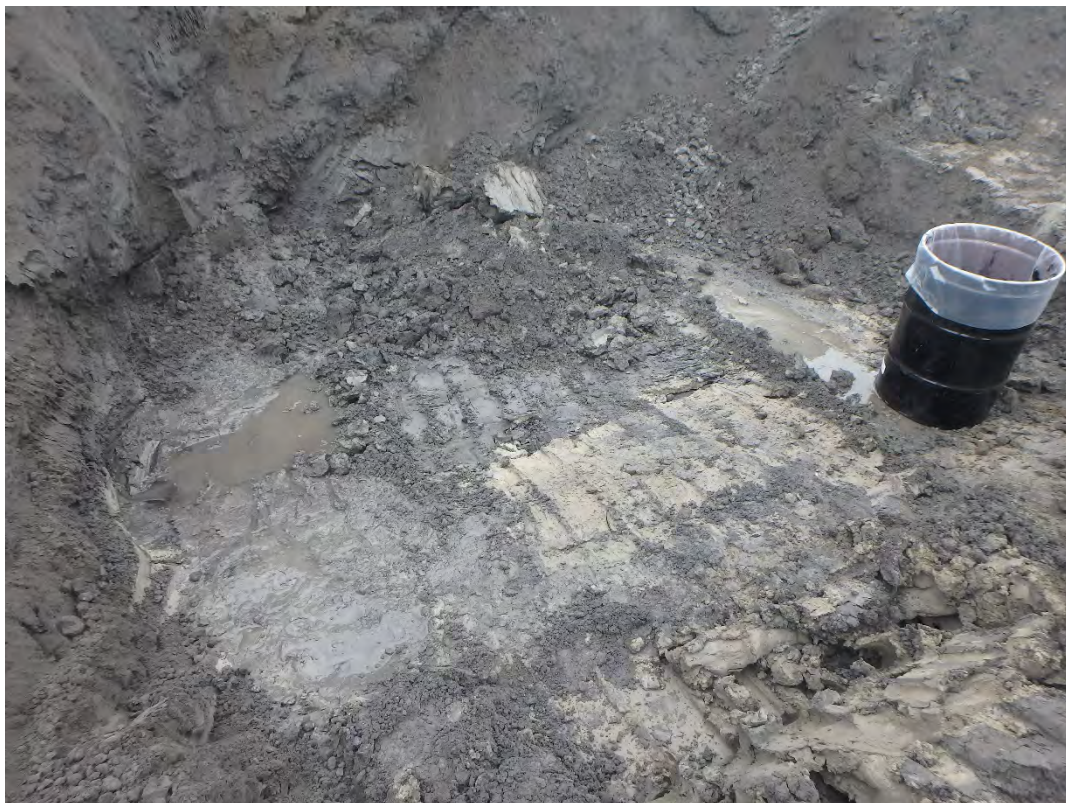
Area that the pool of oil/tar like matter soils after removal and placed in lined 55 gallon drum.
