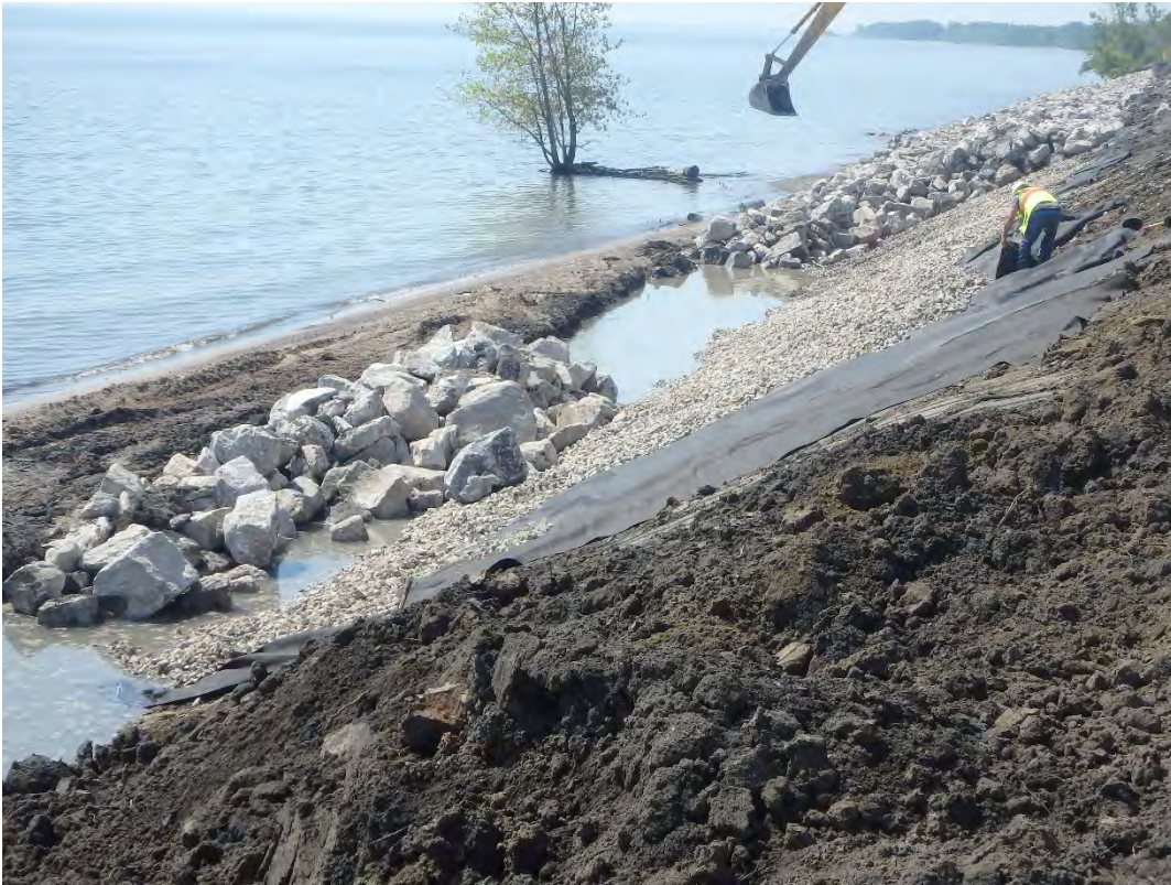
Placement of textile, 2 inch cushion material and 30 inch riprap along shoreline, looking south.
