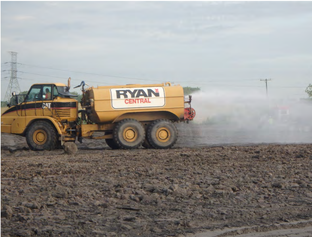
Water truck used to moisture conditioning of placed structural fill and dust control, looking west.
