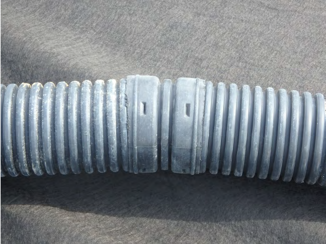
Non-perforated ADS pipe connection on above-cap drain pipe in Pond 1.
