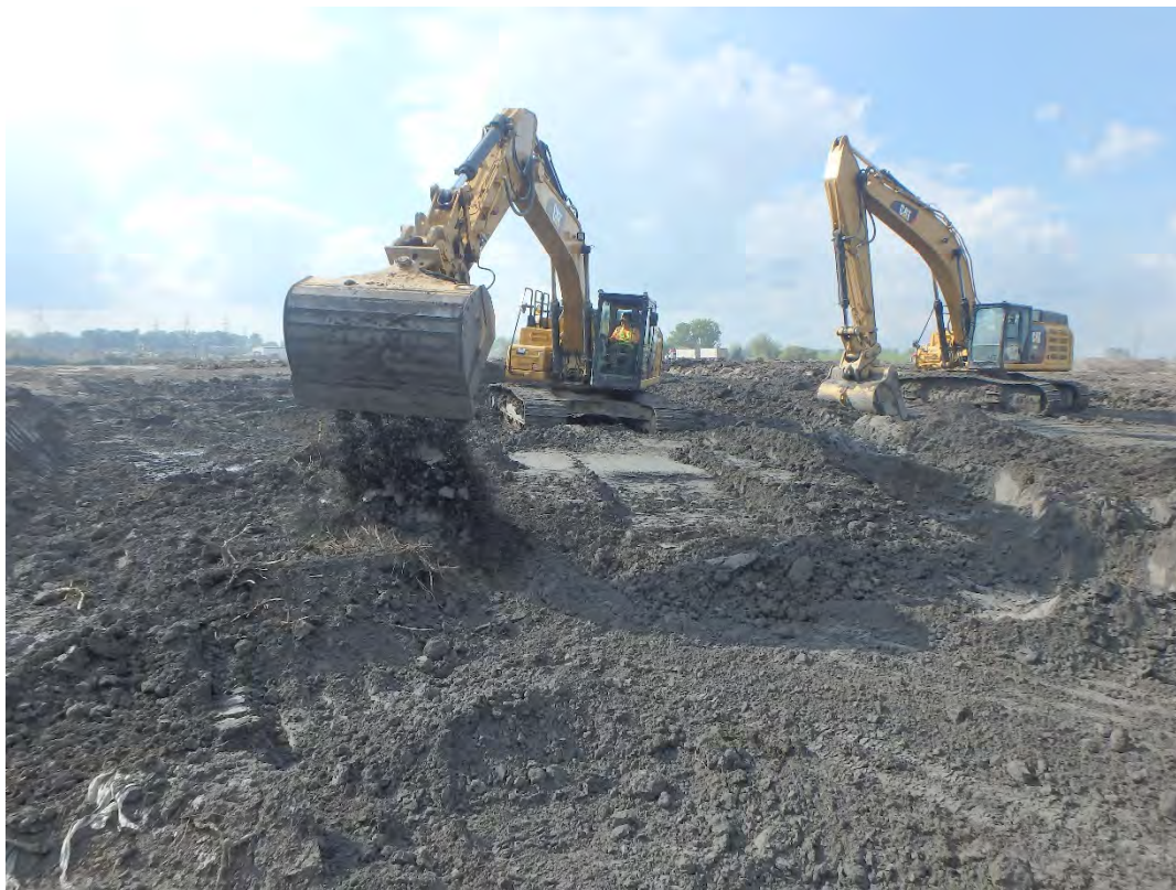
Placing CCR in sump area of Pond 2 for bridging layer, looking northwest.
