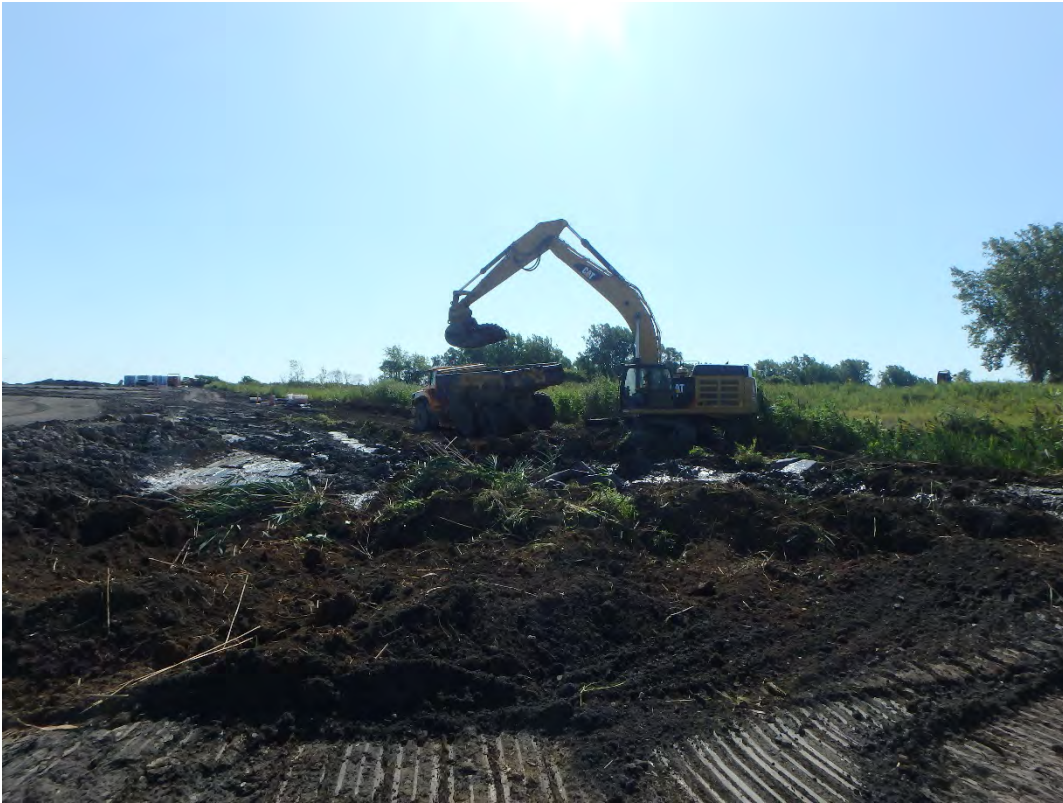
Excavating CCR from area between Pond 2's southwest corner and Fore Bay, looking south.
