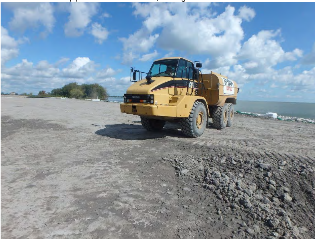
Proof roll of bridging layer in southeast corner of Pond 2, looking northeast.
