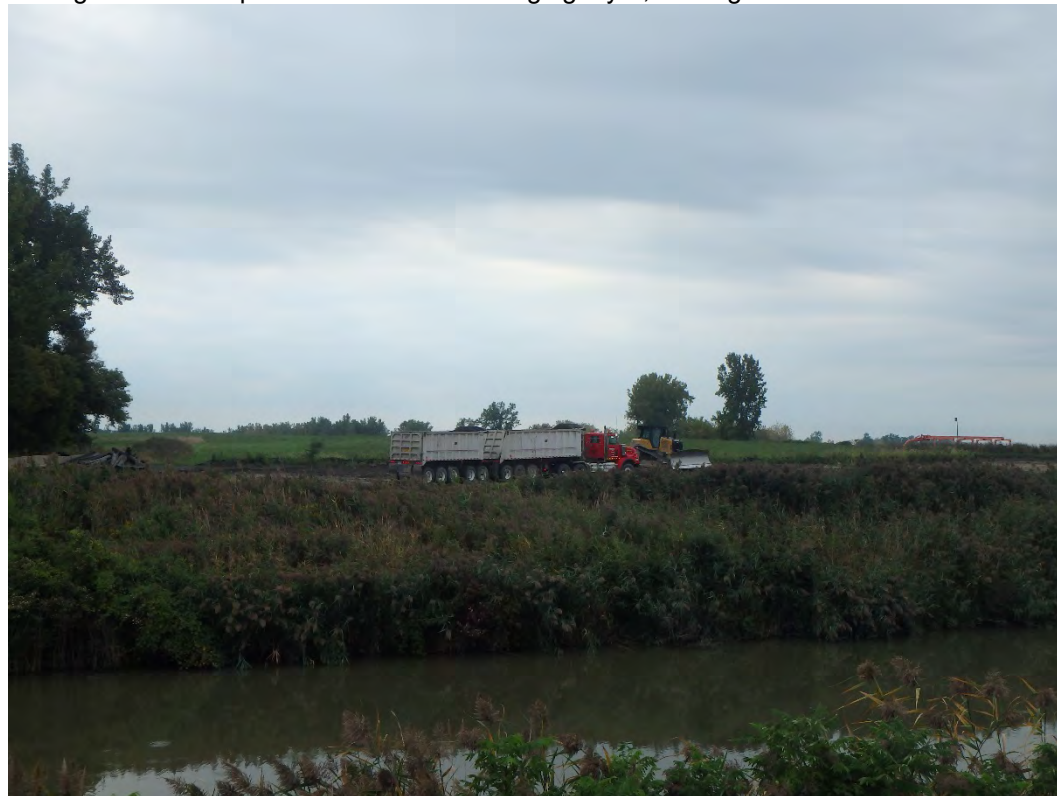
Structural fill being placed in the Chemical Ponds work area, looking south.
