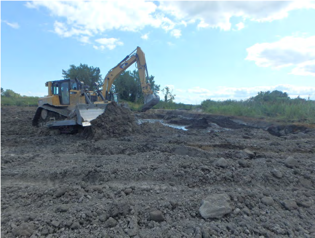
Installing clay cap over cut west of Pond 2 along the fore bay, looking south.
