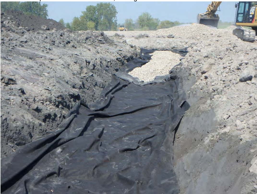
Placing 1x3 inch stone in trench excavated in southeast corner of Pond 2's bridging layer, looking north.
