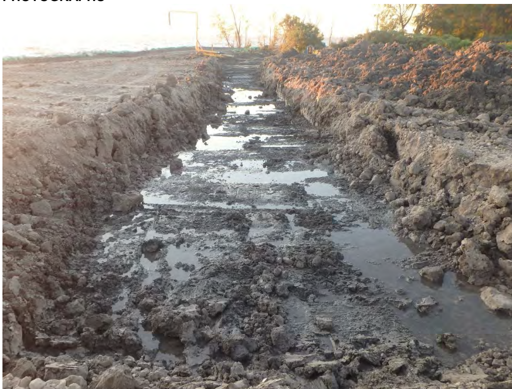
Trench excavated in southeast corner of Pond 2's bridging layer, looking southeast.
