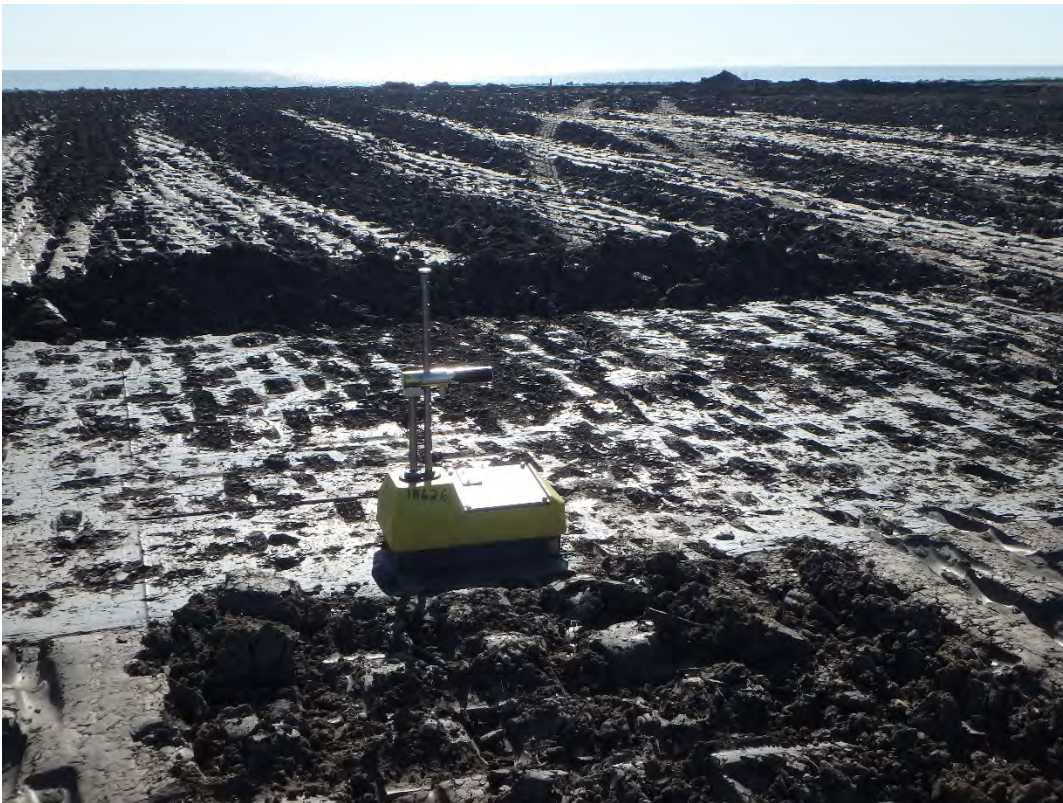
Density testing of placed and compacted structural fill lift in Pond 2, looking east.
