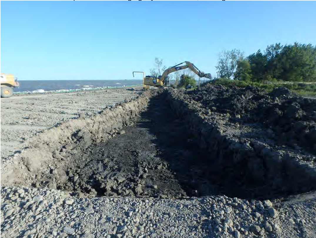
Excavating area of bridging layer in Pond 2 that failed proof roll, looking southeast.
