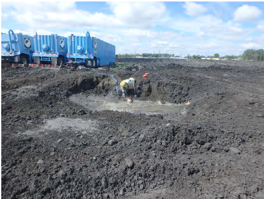
Pumping standing water from southeast corner of Pond 2 into baker tank, looking west.
