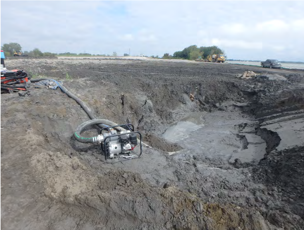
Pumping of standing water from southeast corner of Pond 2 to baker tank, looking northeast.
