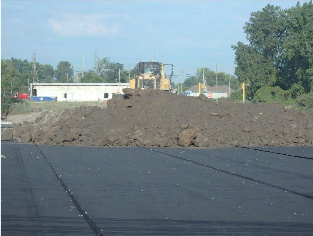
Placement of protective cover for construction of 4 foot haul road in Pond 1, looking west.
