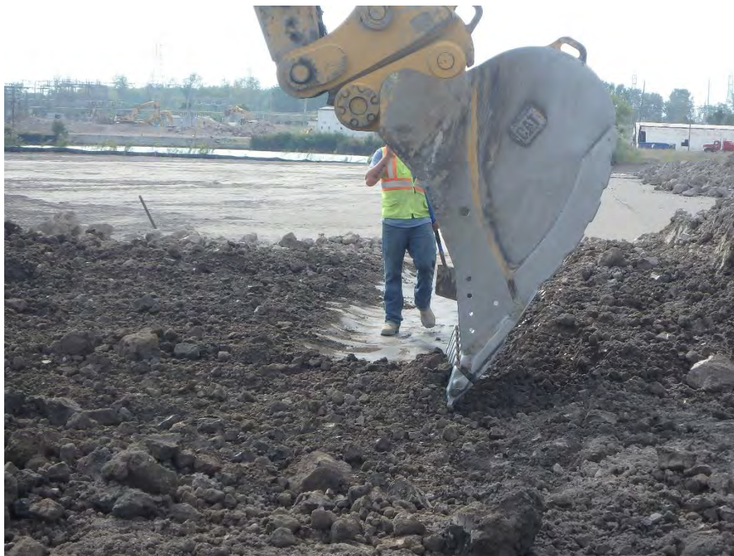
Removing temp ramp atop liner tie-in along south side into Pond 1, looking west.
