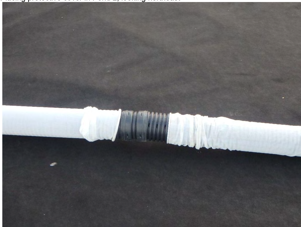
Above-Cap drain pipe with sock
