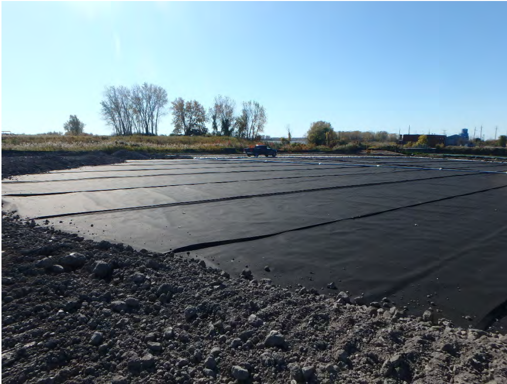
Overview of remaining area of Pond 2 to be covered with protective cover, looking southwest
