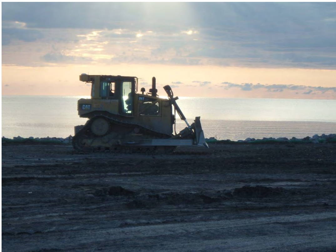
Placement of structural fill outside of Pond 2's southeast corner, looking east.
