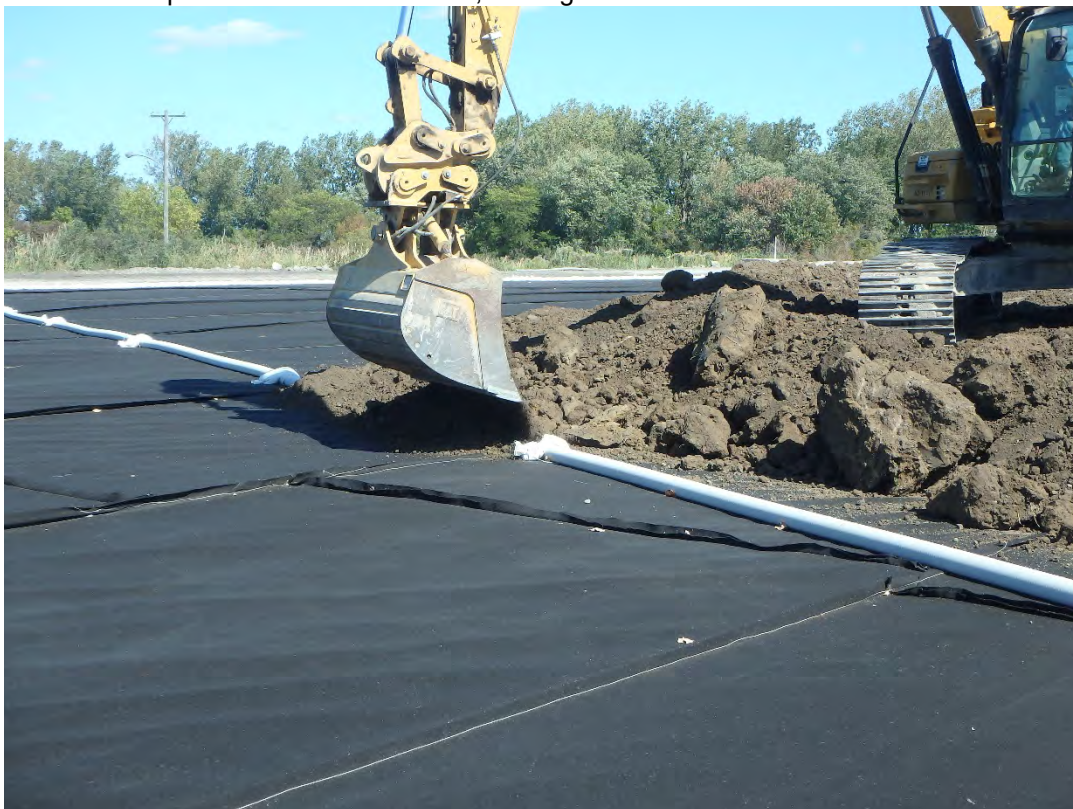
Placement of protective cover over the above-cap drain pipe in Pond 1, looking northeast.
