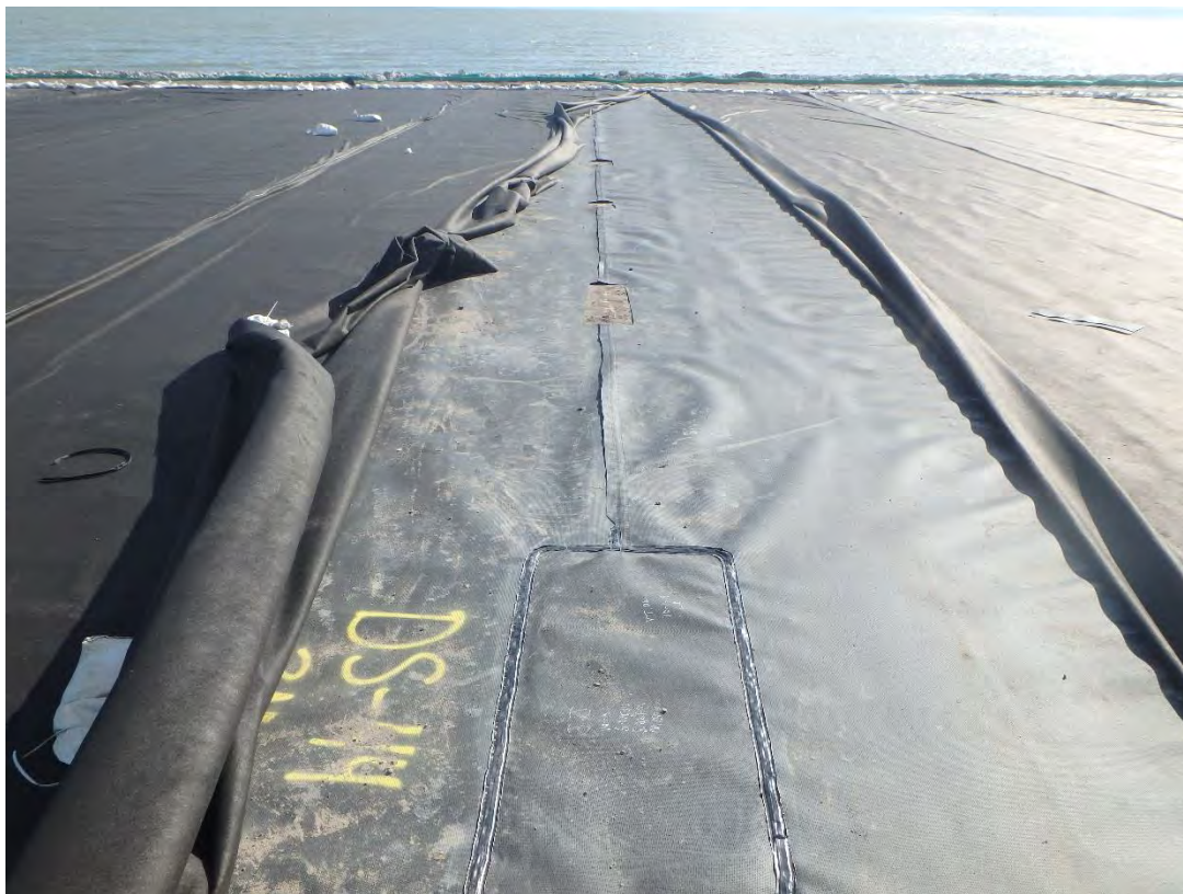
Tracking of failed destructive test seam for capping, looking east
