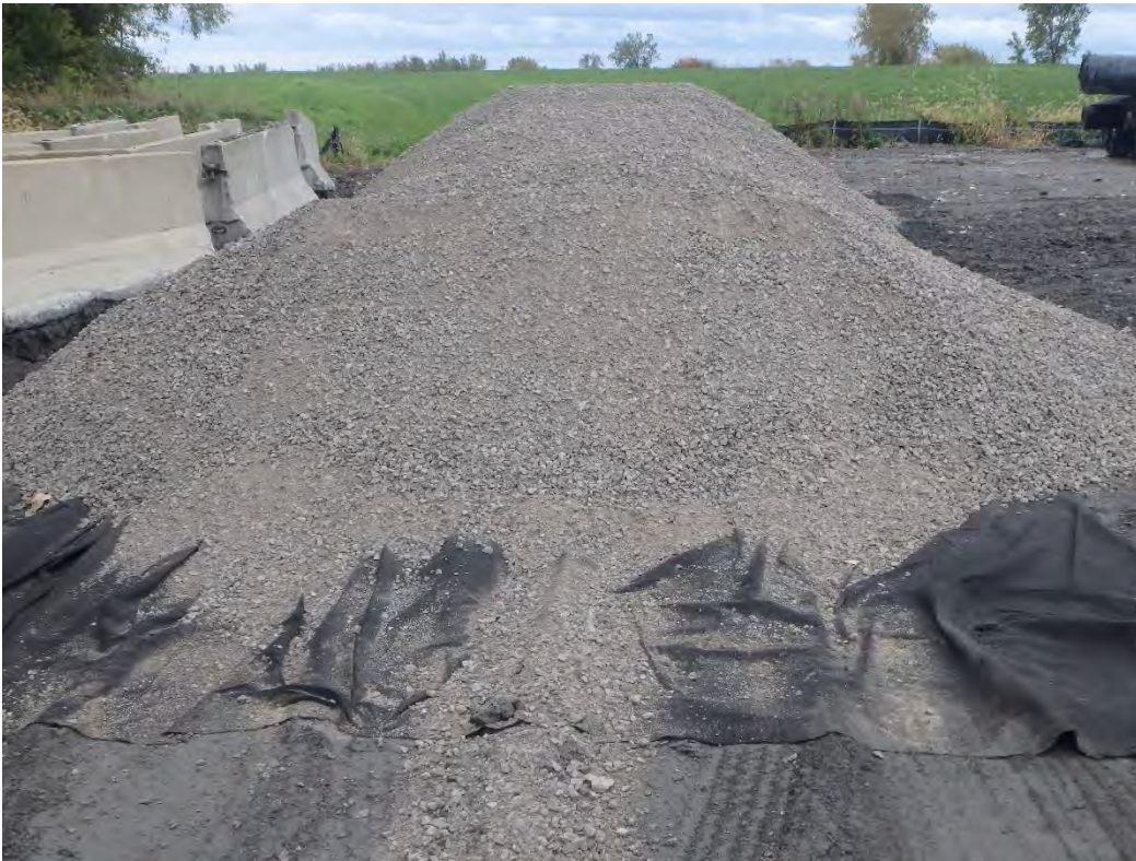
23A imported stone for access road placed atop 10 oz. textile in chemical ponds, looking south
