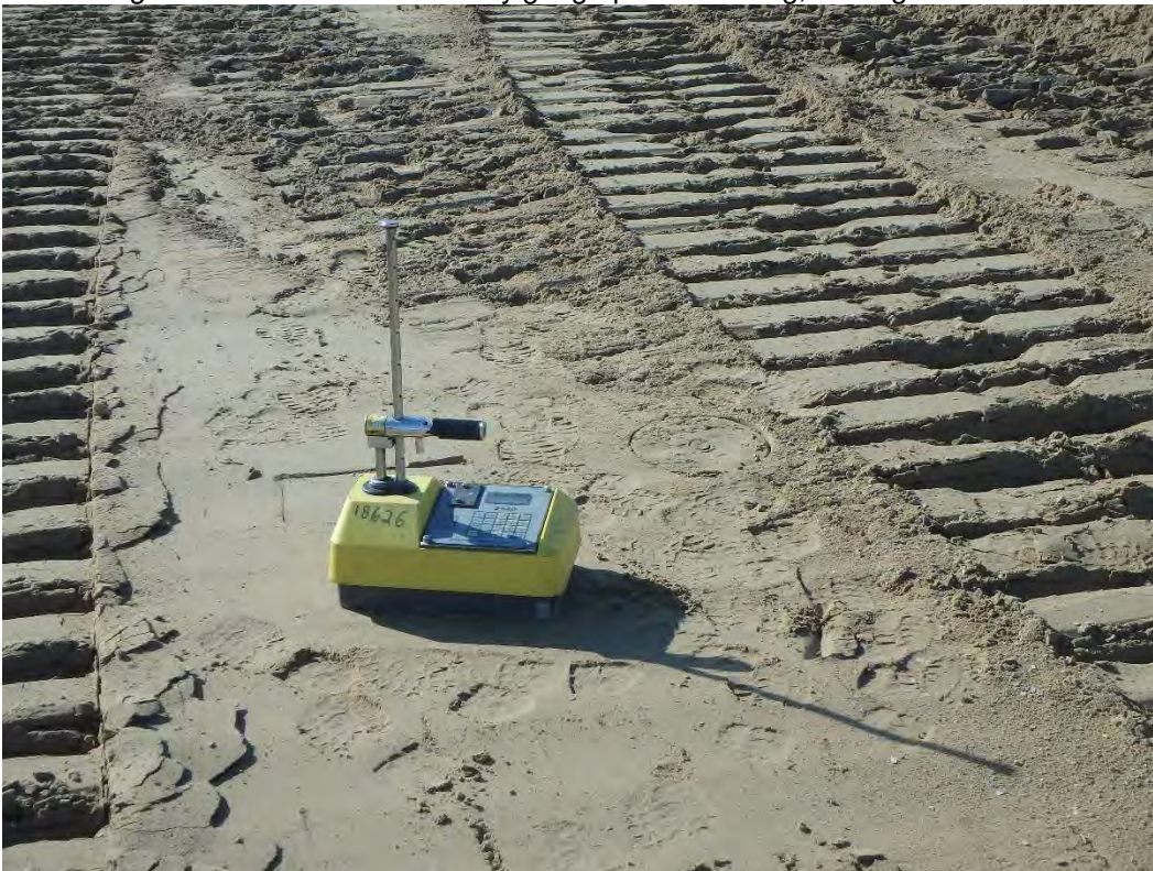
Density test of class II sand placed and compacted for east access road, looking north
