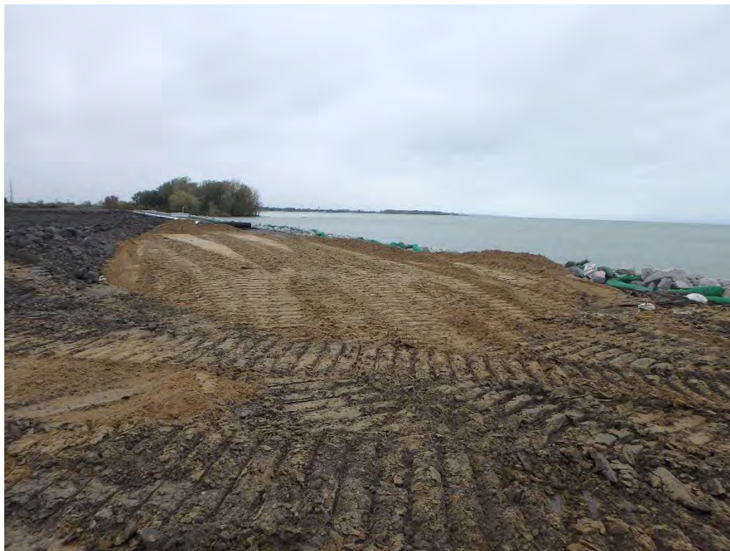
Class II sand imported for access road, looking north from southeast corner of Pond 2
