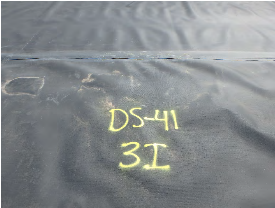
Destructive test and defect number.
