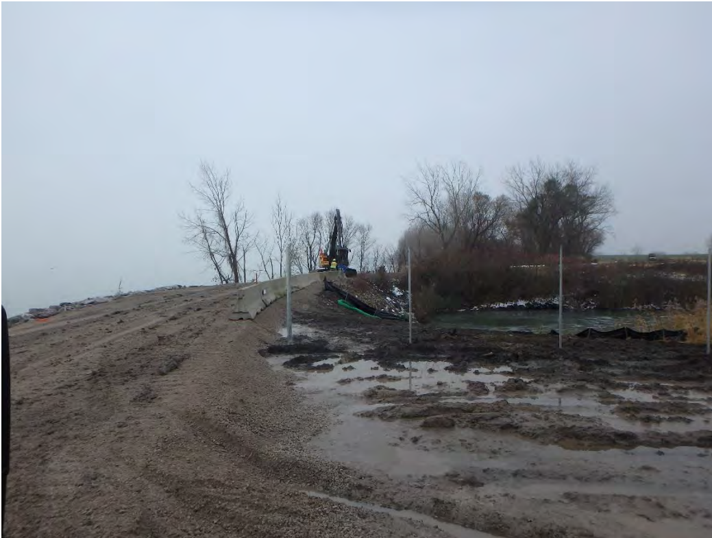
Installing Jersey barriers around horseshoe between Pond 2 and Chemical Pond, looking south
