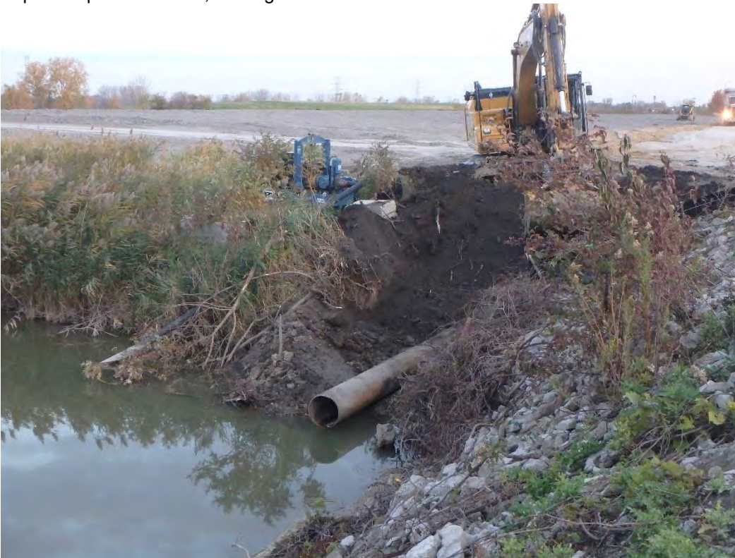
24 inch steel pipe discovered in the northeast corner of the discharge channel, looking north
