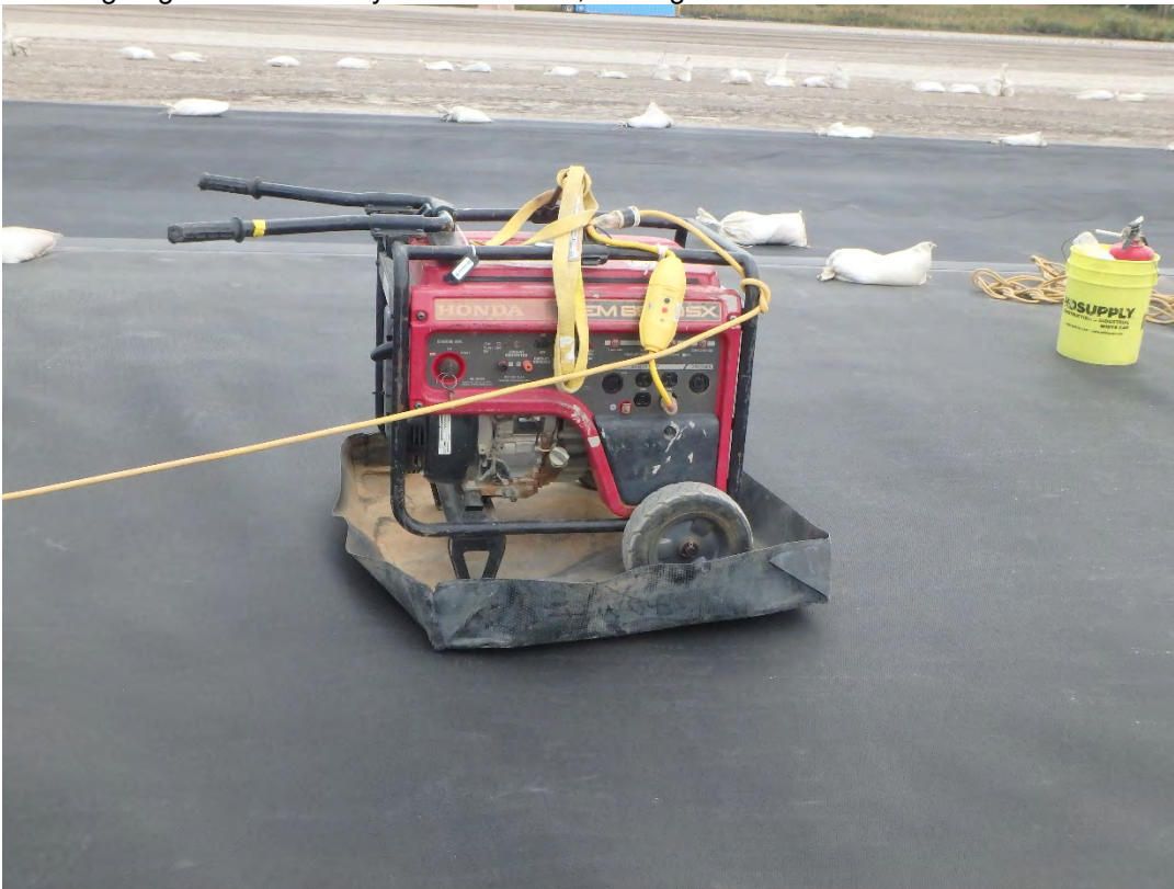
Rub sheet/Tub for generators while on liner, looking south.
