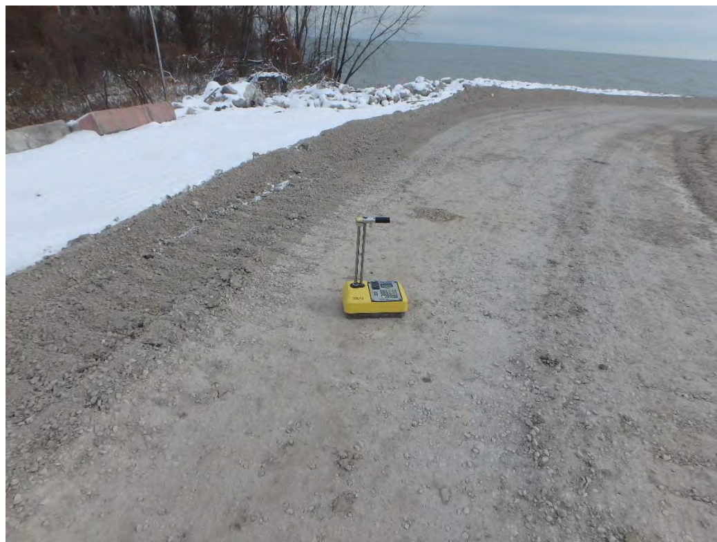
Density testing of road base material for north access road, looking east
