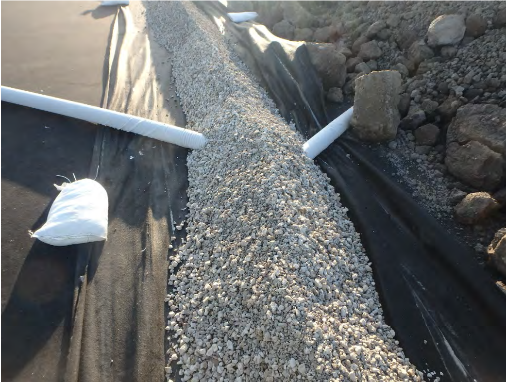
6AA placed around the solid above-cap drain pipe in Pond 1, looking east.
