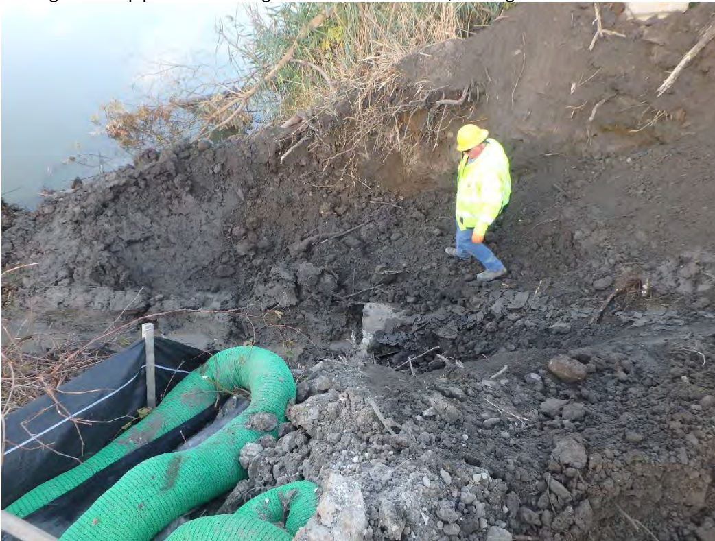
End of 24 inch pipe from discharge channel to be capped, looking west
