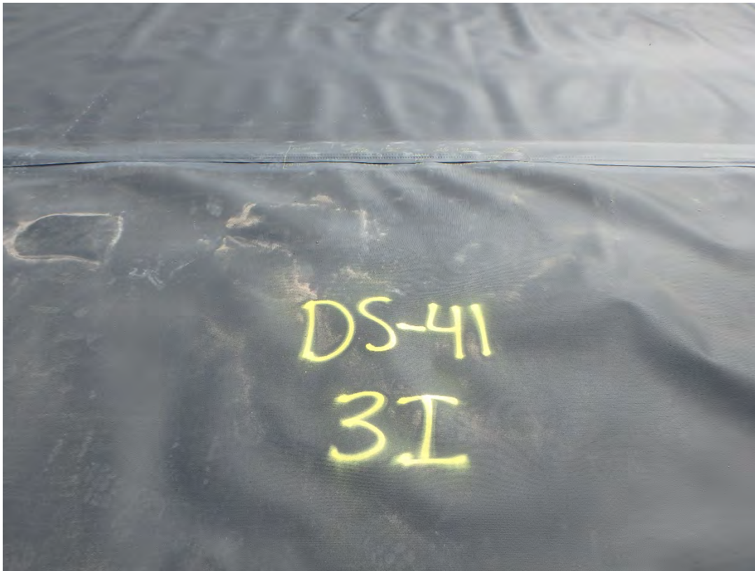
Destructive test and defect number.
