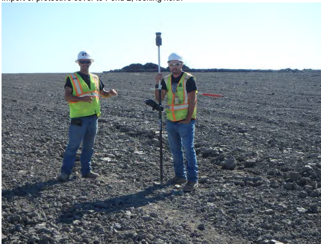
Rowe shooting protective cover placed in Pond 1, looking east
