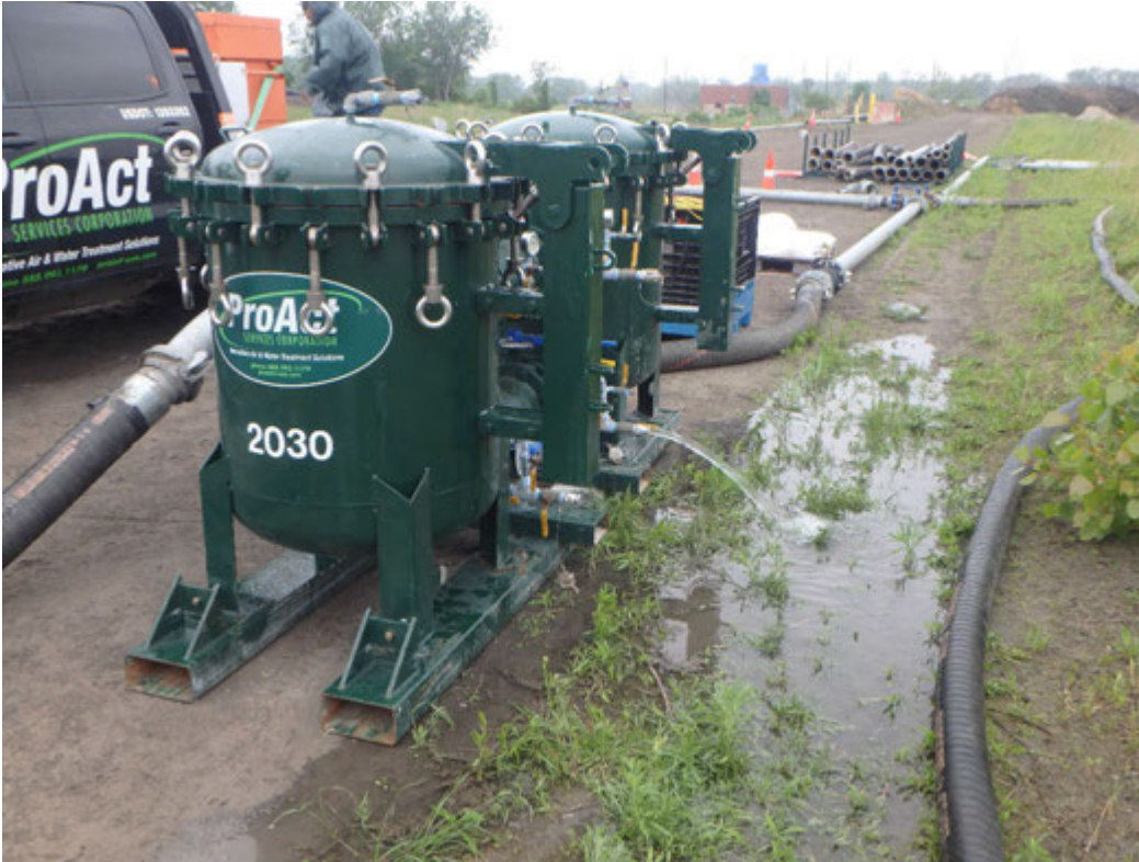
Backflush of dewatering system at Pond 2, looking west.
