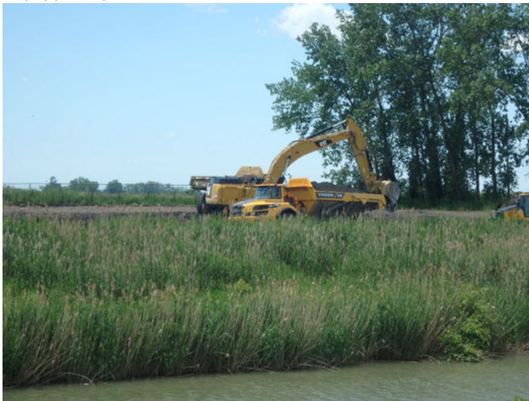
Cutting down Chemical Pond A to 2 feet below final grade, looking south.
