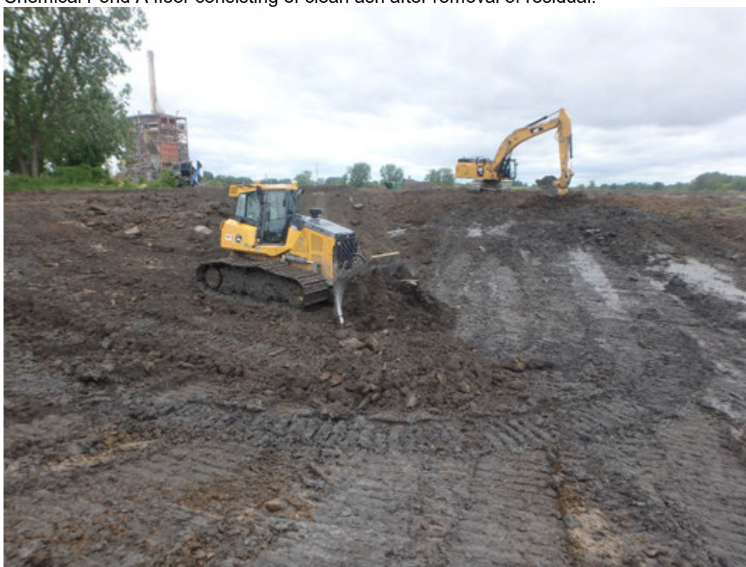
Placing bridging layer of structural fill across floor of Chemical Pond A, Looking North.
