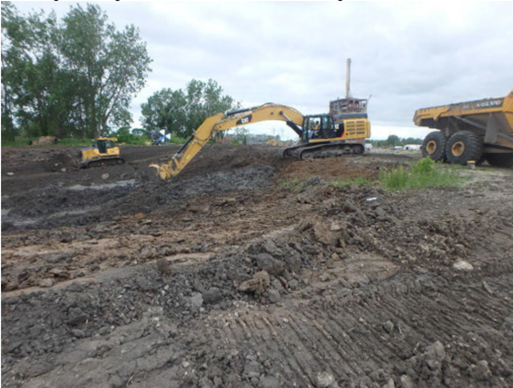
Loadout of residual from Chemical Pond A for transport to Pond 1, Looking West.
