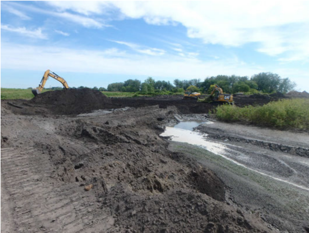
Removing north perimeter road, material to be used for bridging layer. Looking Northeast.
