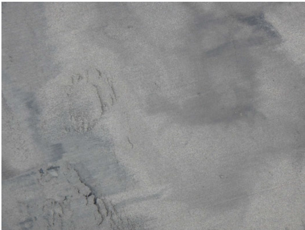
Chemical Pond A floor consisting of clean ash after removal of residual.
