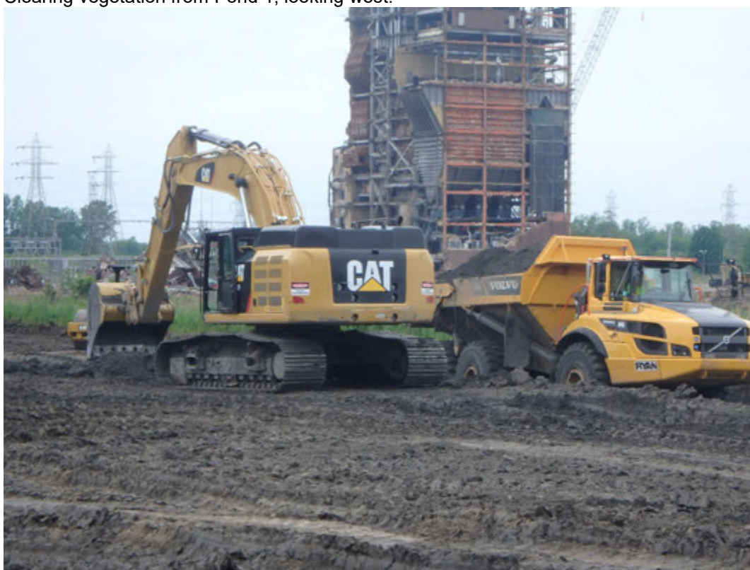
Cutting area north of Chemical Pond B down to structural fill grade, looking west.
