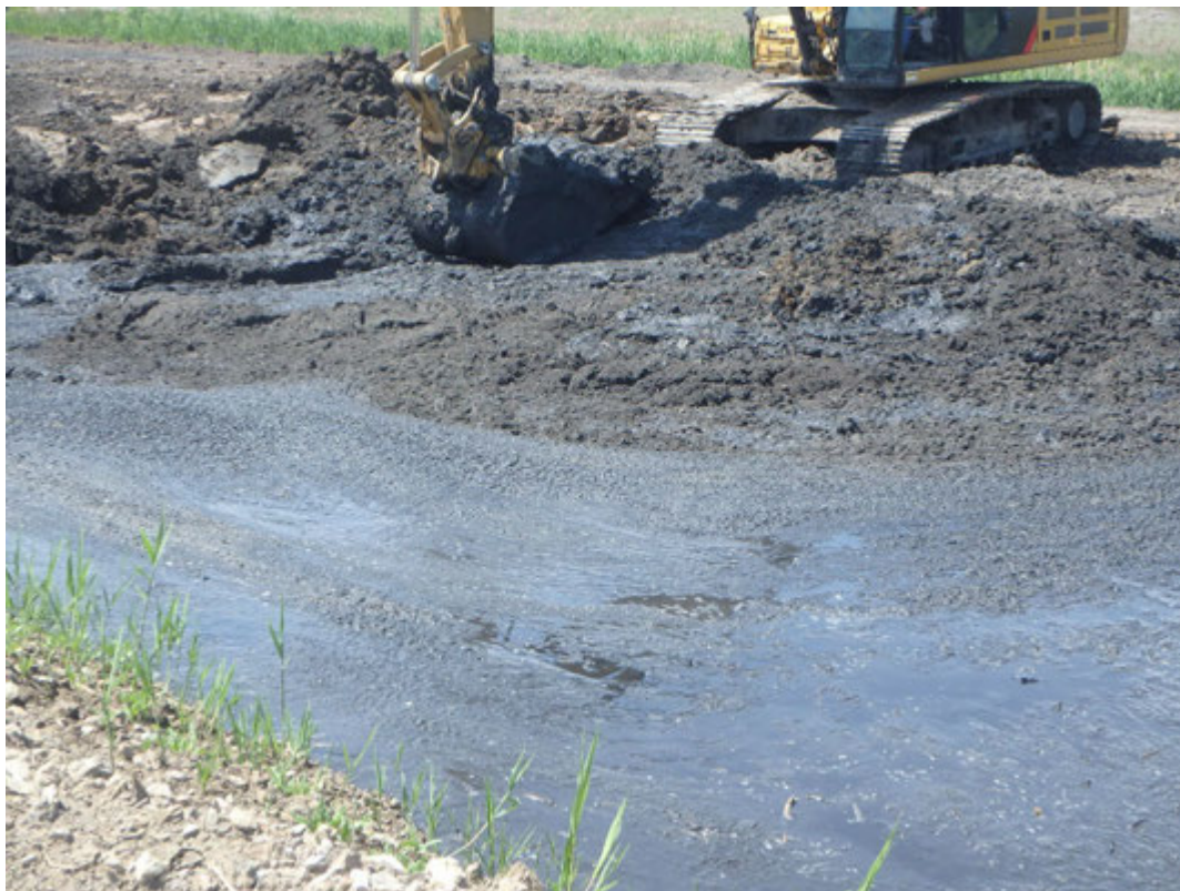
Mixing berm material with pond residuals to dry for transport to Pond 1, Looking north.
