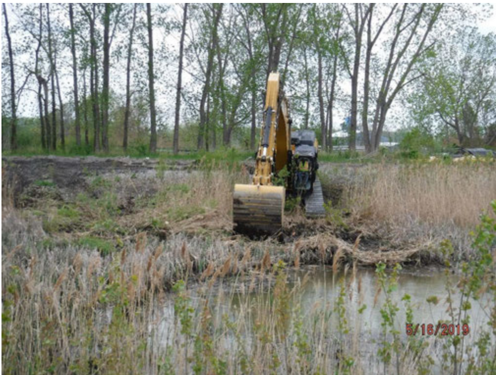
Chemical Pond A work to force water into northeast corner to enable dewatering into Chemical Pond B.
