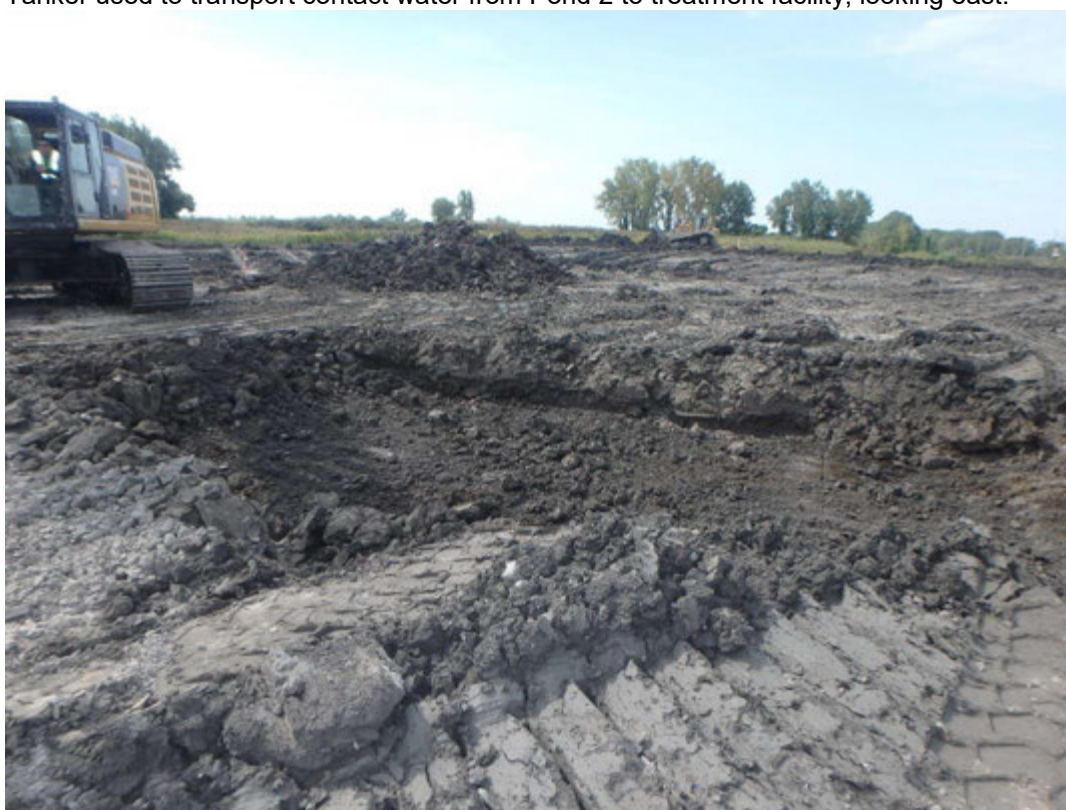
Soft spot excavated in Pond 2 bridging layer, looking southwest.
