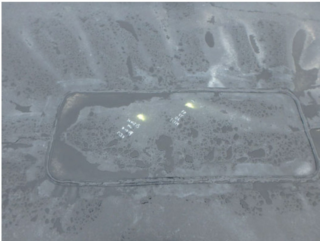
Repaired and vacuum tested defect.
