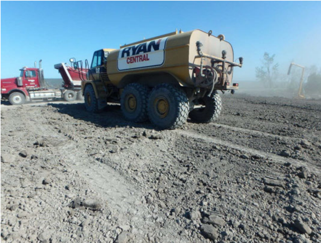
Water truck used for proof roll of bridging layer in Pond 2, looking east.
