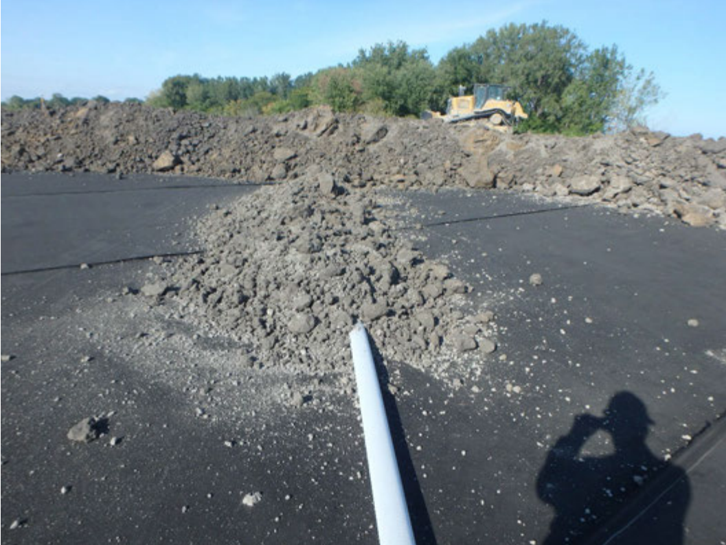
Protective cover placed atop the 4 inch ADS perforated drain pipe in Pond 1, looking northeast.
