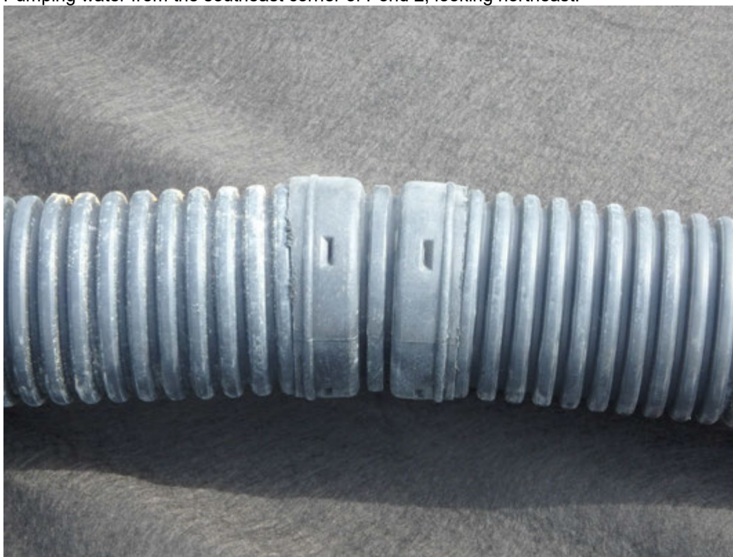
Non-perforated ADS pipe connection on above-cap drain pipe in Pond 1.
