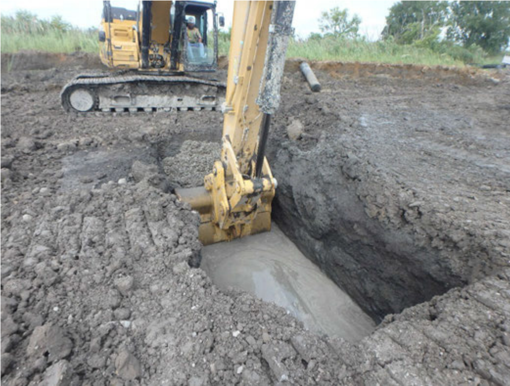
Excavation of French Drain trench to remove drainage stone and install clay plug, looking west.
