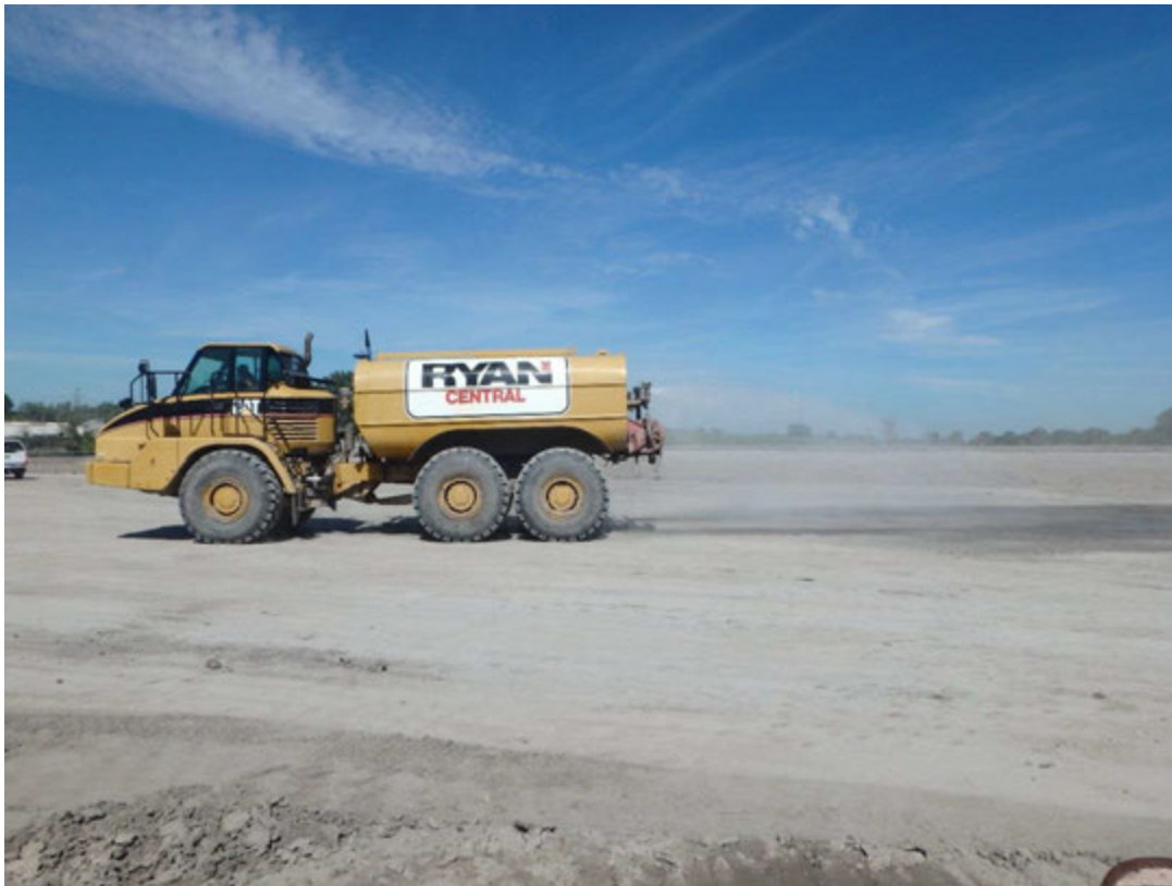
Water truck used for dust control and moisture conditioning of prepared sub-grade, looking north.
