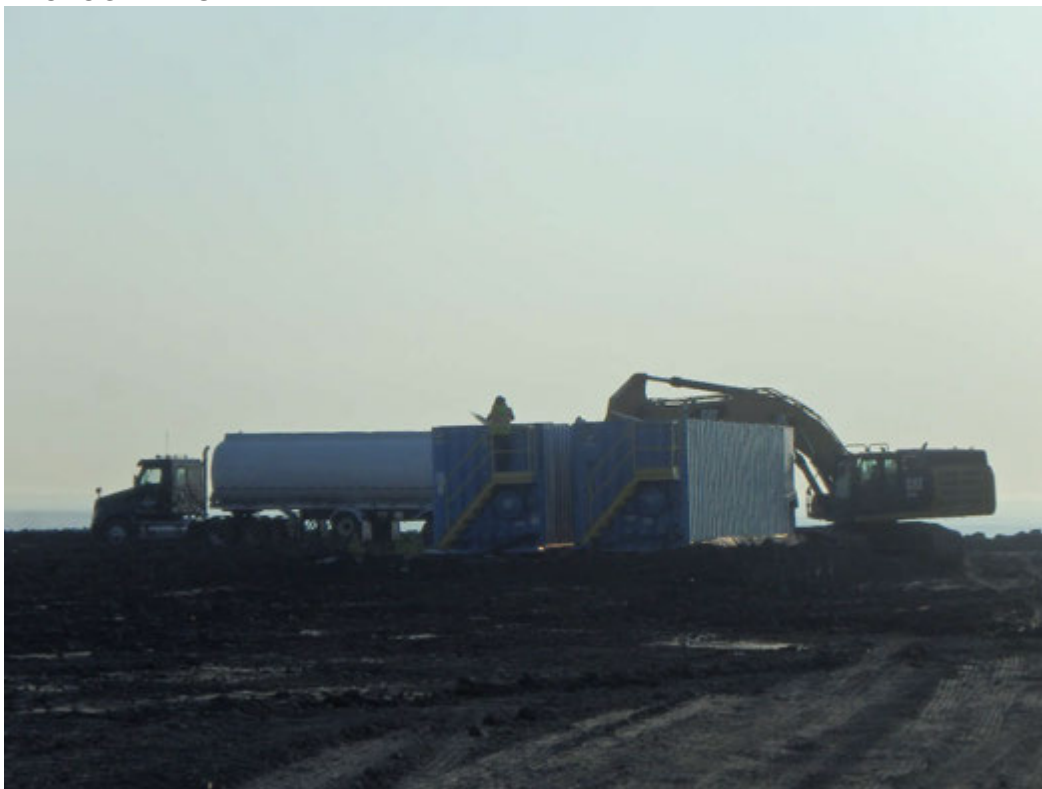
Pumping baker tanks into tanker for transport to treatment facility, looking east.
