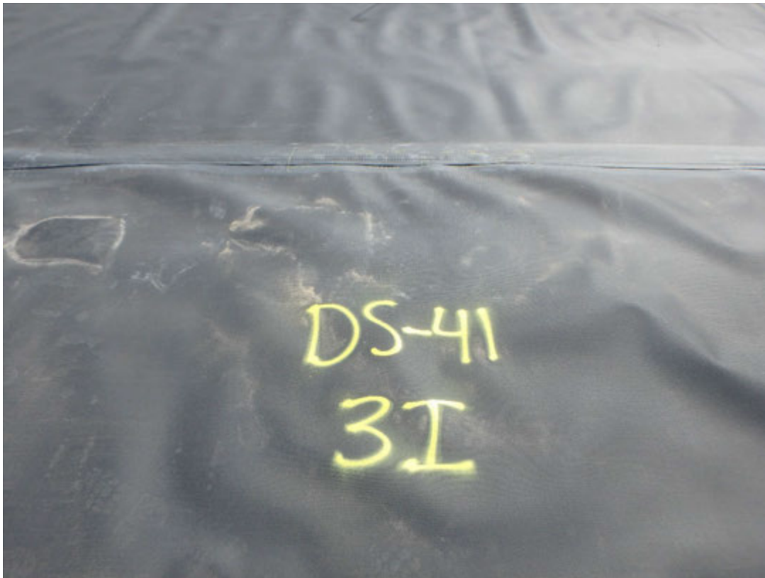
Destructive test and defect number.
