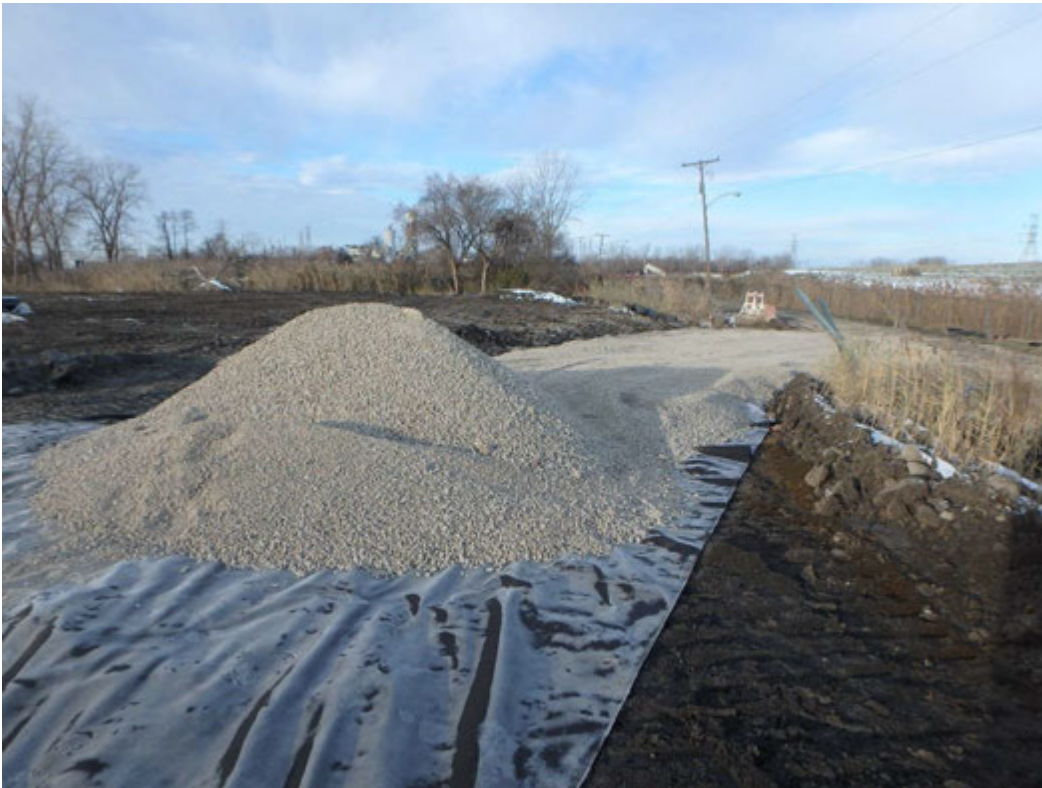
Placing 8 inch lift of 21AA for access ramps asphalt base, looking northwest
