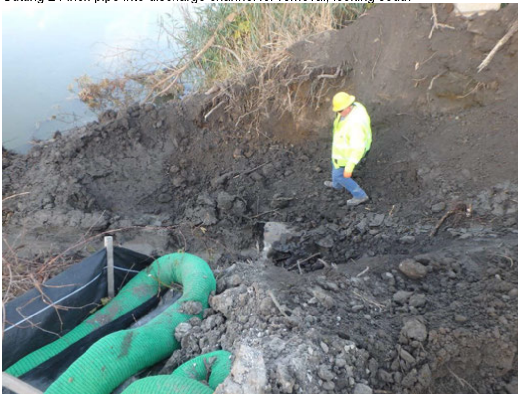
End of 24 inch pipe from discharge channel to be capped, looking west
