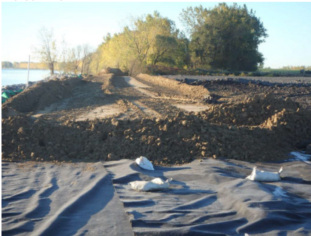
Class II placed for east access road sub-base east of Pond 2, looking south
