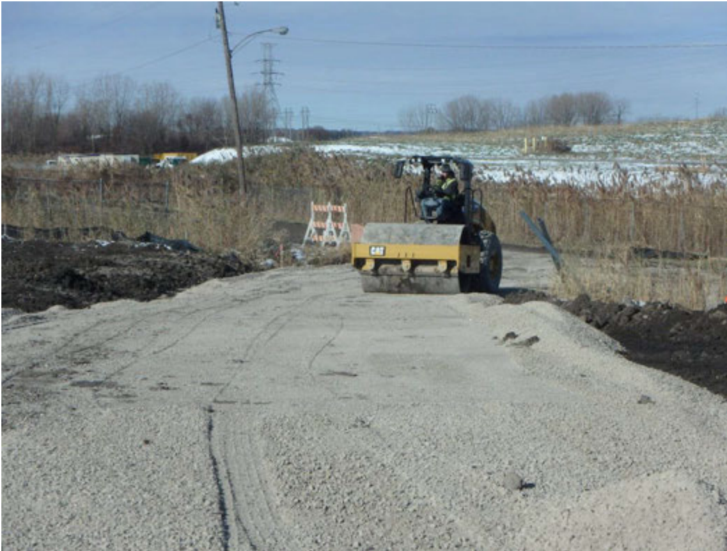
Compacting 21AA placed for access ramp using smooth drum roller, looking north
