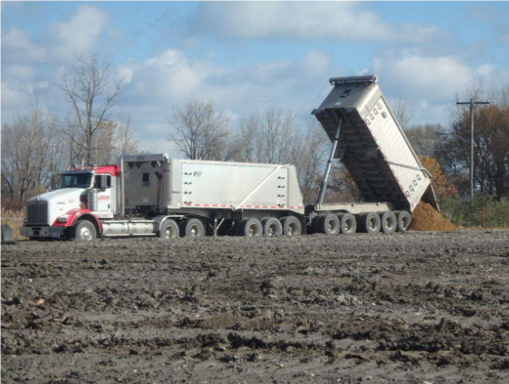
Import of Class II/III sand for north access road sub-base, looking northeast
