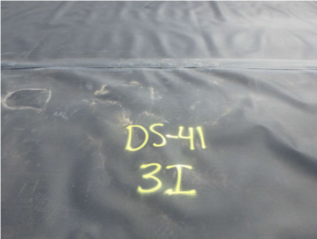
Destructive test and defect number.
