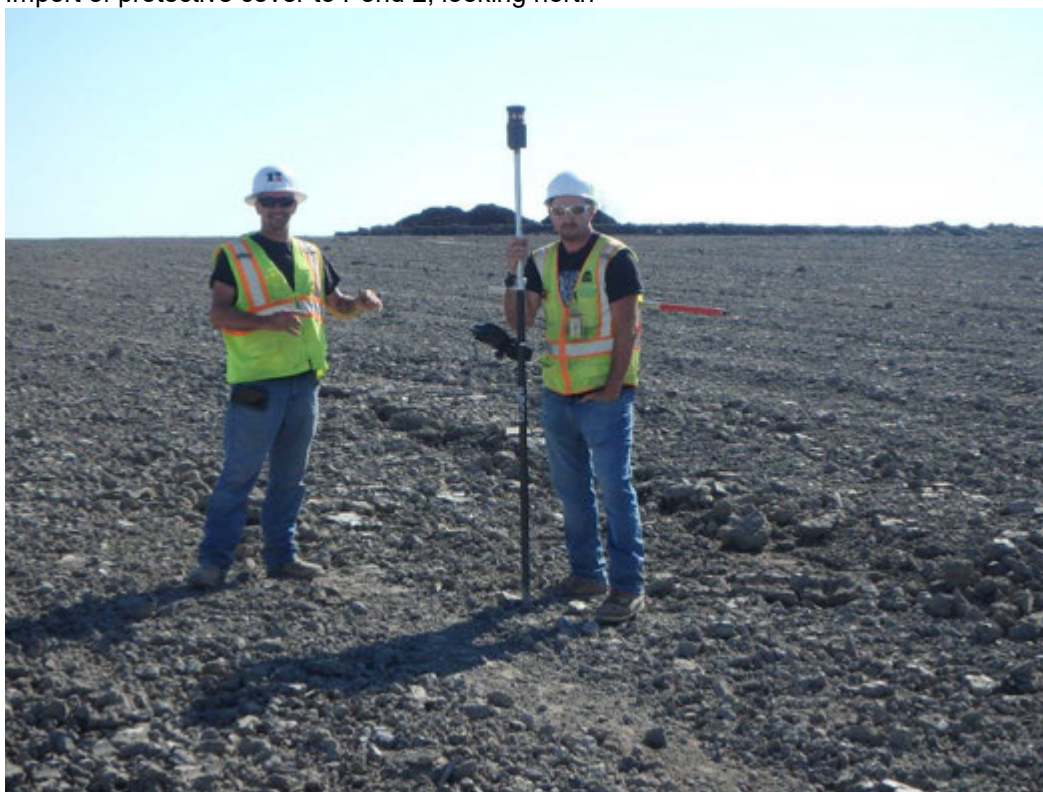
Rowe shooting protective cover placed in Pond 1, looking east
